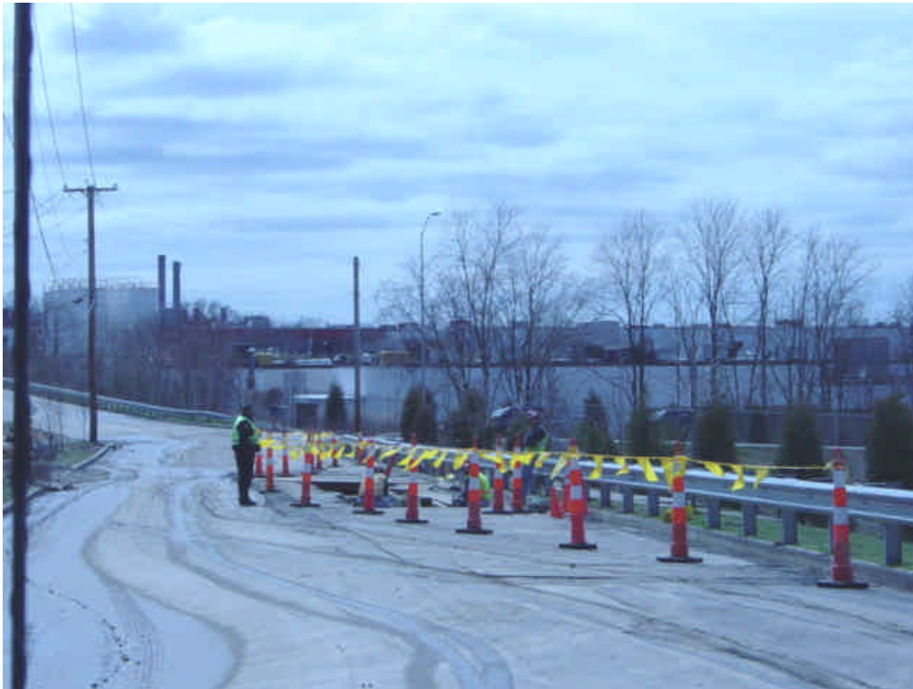
Photo of trenching activities at sta. #1096 near the Milford lay-down yard. The roadway appears to have been swept recently.
