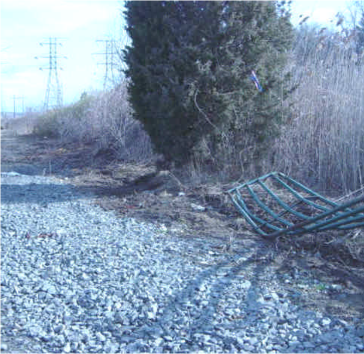
Photo taken of sta. #1053 where the silt fence in disrepair has been removed along with the materials previously noted in the wetland (including metal gate). It appears that Segment 3 work in the cross-country area is complete for now.
