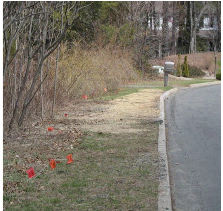
View of an area off Old Farms Rd. which was regraded, seeded, and mulched to provide temporary stabilization until grass establishes.
