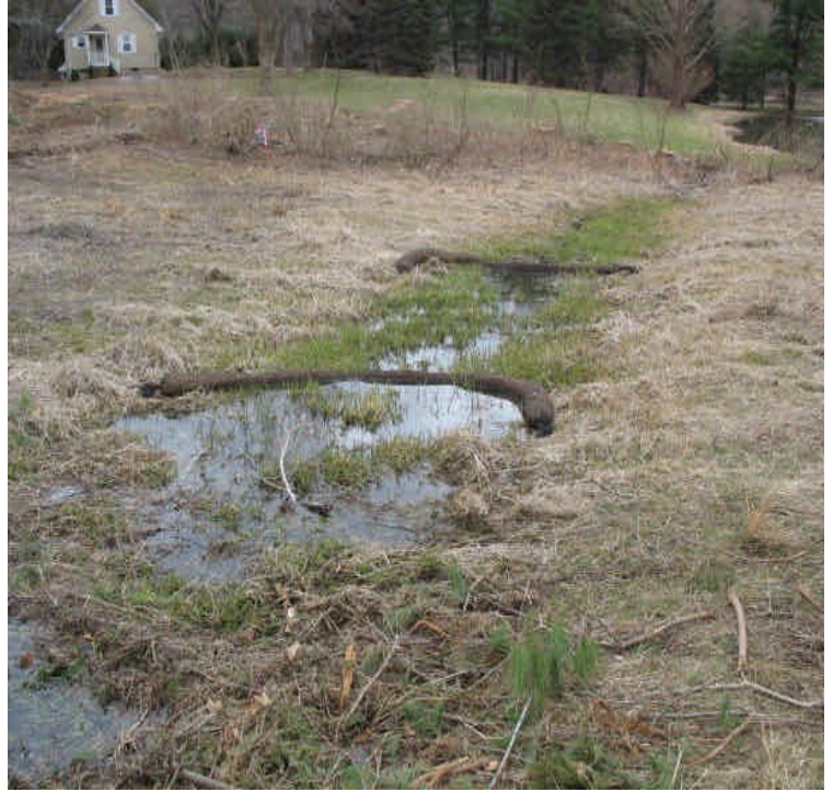
Filter socks were added downgradient of the work off Liney Hall Ln. No turbidity issues were noted.
