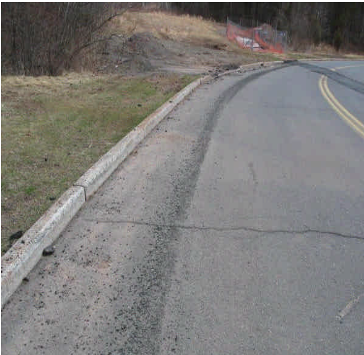
The trench was patched along Old Farms Rd. Some loose asphalt or "crumbling" was noted along the edge of the roadway. In the background, safety fence remains around the transition pit and an area of adjacent exposed soil and leftover fill is located in the overhead ROW. Extra material should be removed and the area should be mulched.
