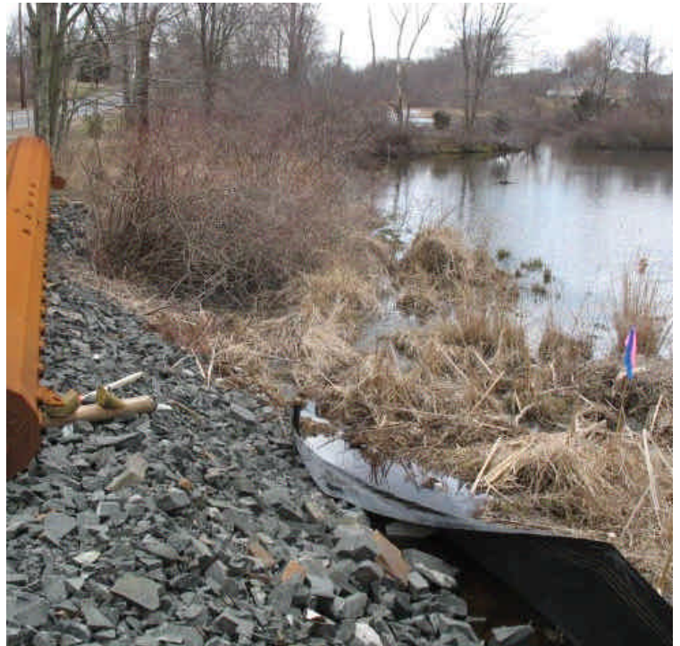
Close-up view of an area where the fence was overwhelmed by the installed stone. Extend controls to keep a visual limit of work in the wetland here.
