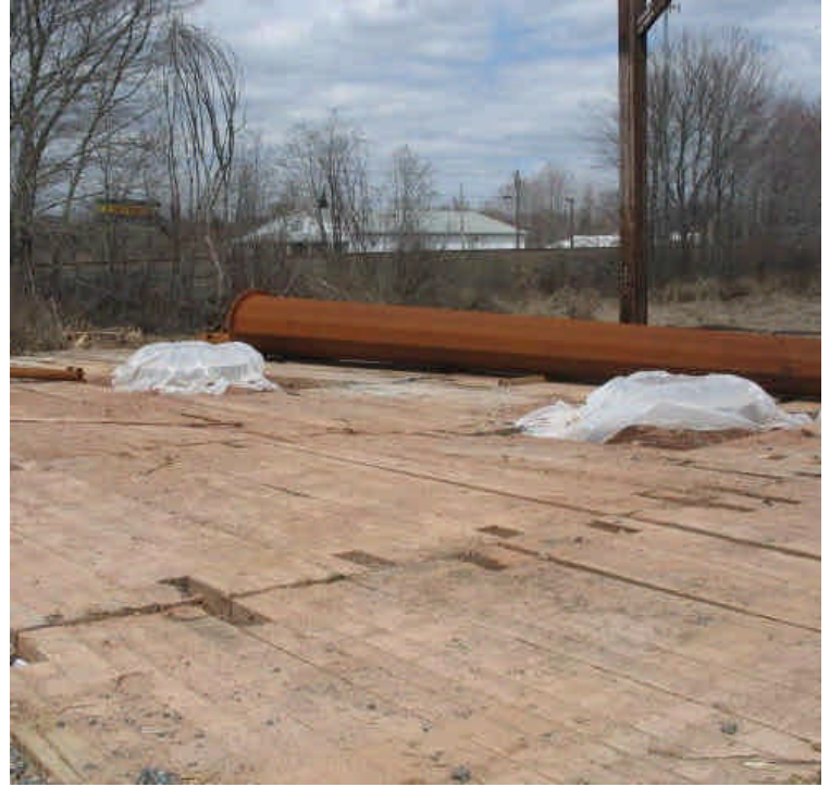
View of timber mat pad constructed off Powers Rd with several completed foundations.
