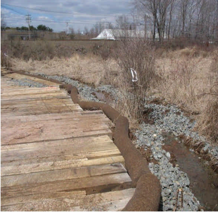
Silt fence removed, filter socks installed for erosion controls off Powers Rd.
