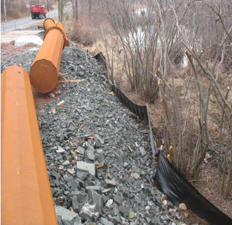
Controls added along wetlands off Woodhouse Ave. Extend and reinforce controls as needed. The stone layers appear to be putting stress on the fence in some spots.
