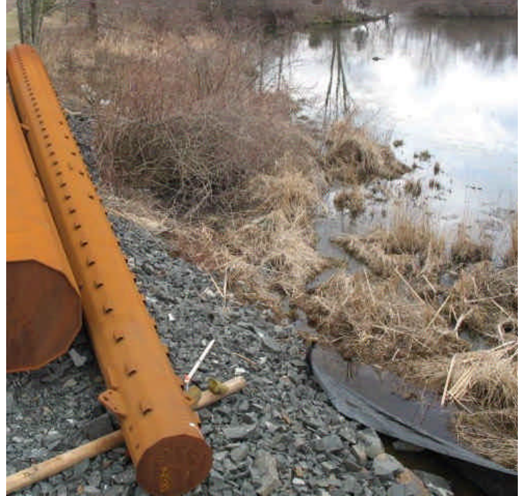
Close-up view of an area where the fence was overwhelmed by the installed stone. Extend controls to keep an approved limit of work in the wetland here.
