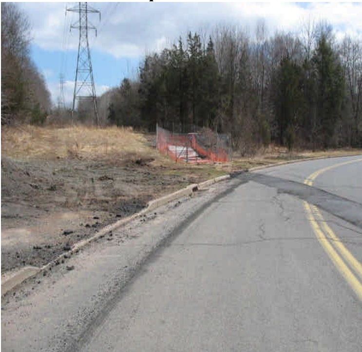
Safety fence remains around the transition pit located off Old Farms Road. An area of adjacent exposed soil and leftover fill is located in the overhead ROW. Extra material should be removed and the area mulched/temporarily stabilized.
