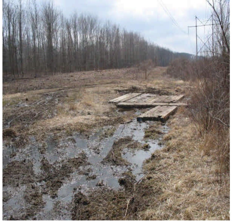
Partial timber mat crossing south of Carpenter Lane for clearing crew. Controls should be added as needed, when work continues.
