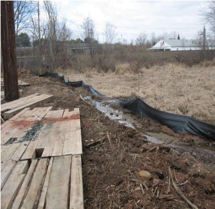
View of timber mats in place for pad construction and erosion controls off Powers Rd
