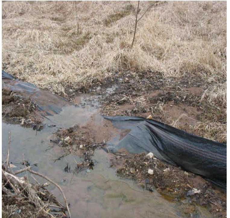
Run-off has washed over a section of silt fence, resulting in minor sedimentation within the wetlands off Powers Rd. Repair the fence as soon as possible to prevent future sediment accumulation.
