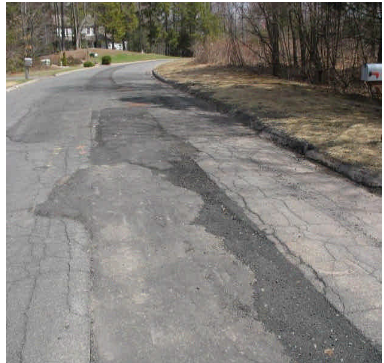
The trench was patched along Old Farms Rd. Some loose asphalt or "crumbling" was noted along the edge of the roadway.
