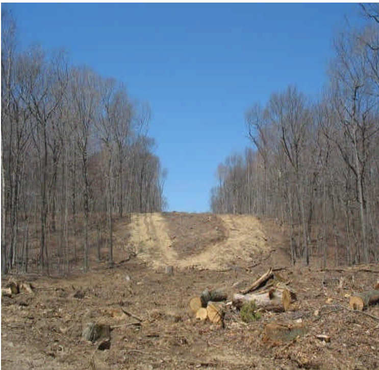
Minor washouts/gullies were noted on the steep slope due to heavy rains last week. Mulch was in place prior to the rain.
