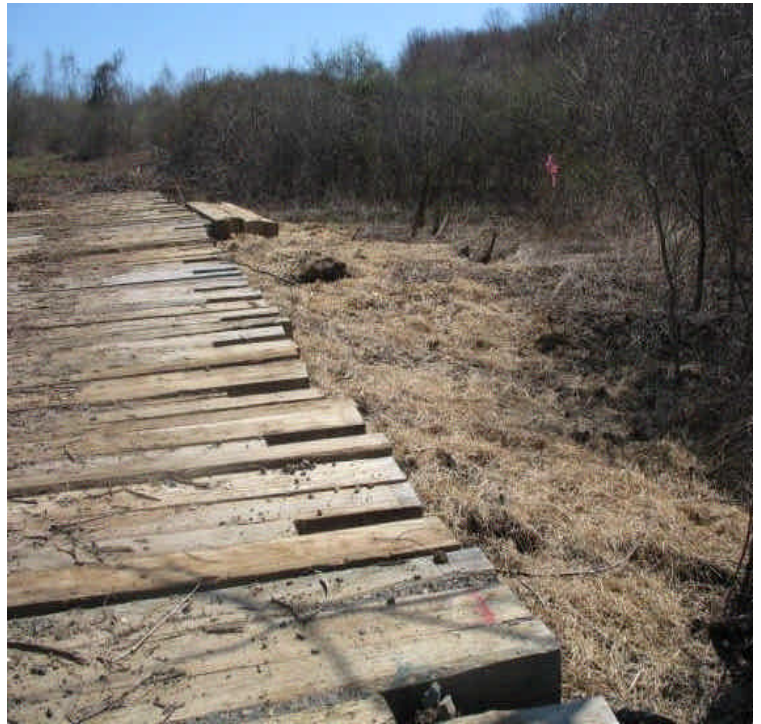
Hay mulch was used along the edge of mats and wetlands near Rte 17 to temporarily stabilize the exposed soil.
