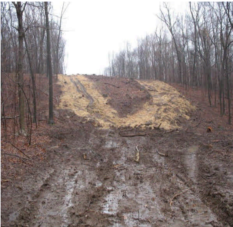
Minor washouts/gullies were noted on the steep slope due to heavy rains.
