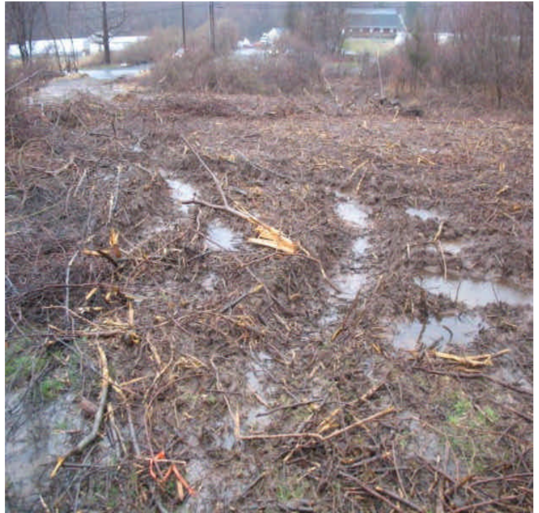
Ruts were observed due to equipment tracking through wetlands near Rte 17. Mats should be installed to support vehicles before they access saturated/wetland areas.
