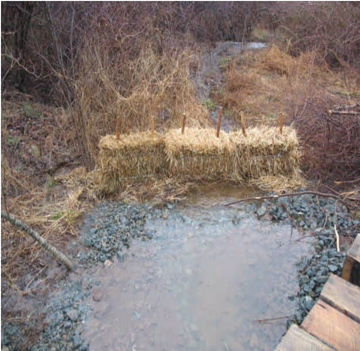
Stormwater controls installed adjacent to the timber mat crossing off Rte 17. Clear water was flowing off site.
