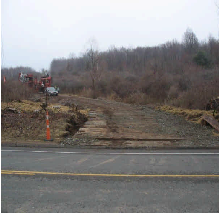
View from the contractor yard, looking across Rte. 17 at the access to the 1b ROW. The access is matted and sediment tracking was not an issue on the roadway.
