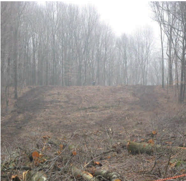
View of the newly cleared ROW looking toward the Black Walnut Dr. area.
