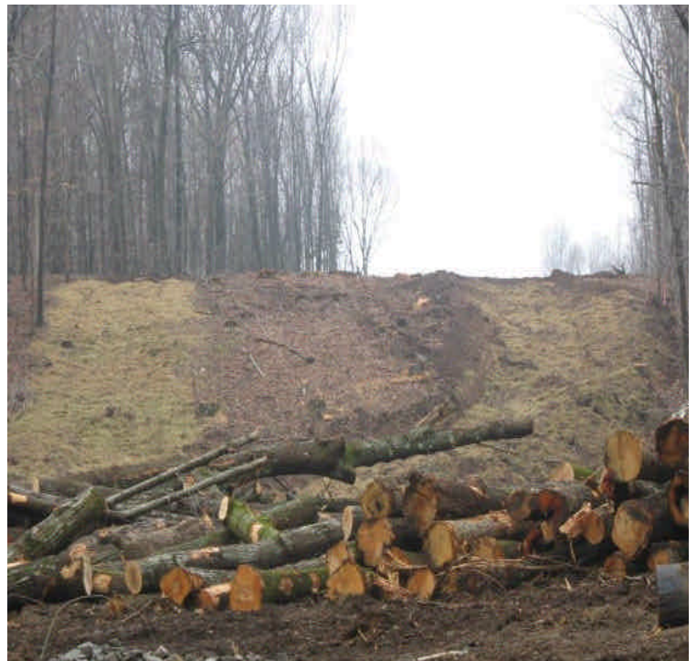
View from the ROW off Black Walnut Dr. Slopes have been mulched to temporarily stabilize the soils.
