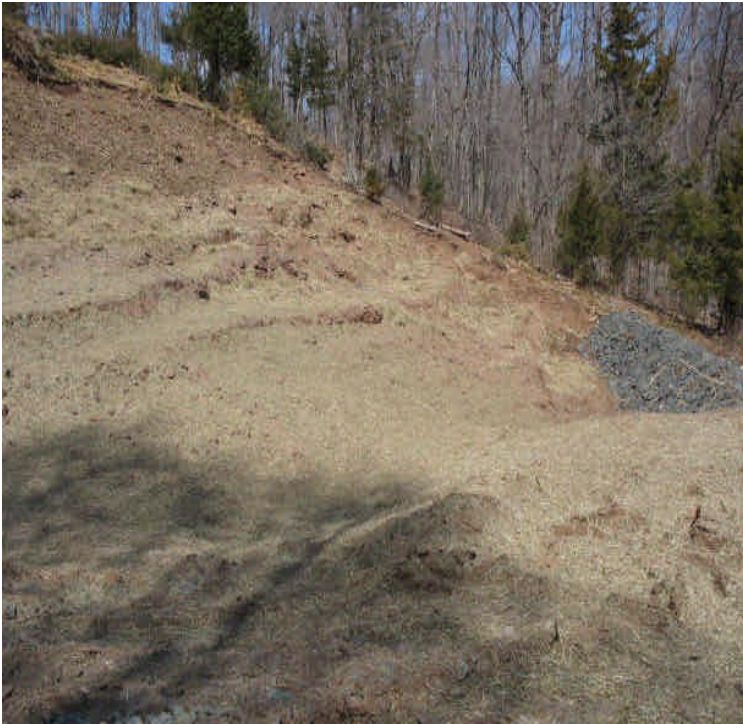
Mulch was placed along slopes off Arbutus St. Stone check dam were also installed to filter run-off.
