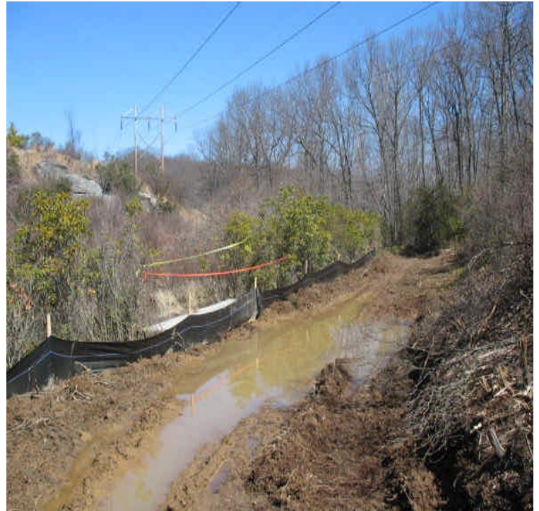
Water has ponded up along the access road in several locations west of Scovill Rock. Disturbance from vehicle tracking could result in turbid run-off. Good controls were installed.
