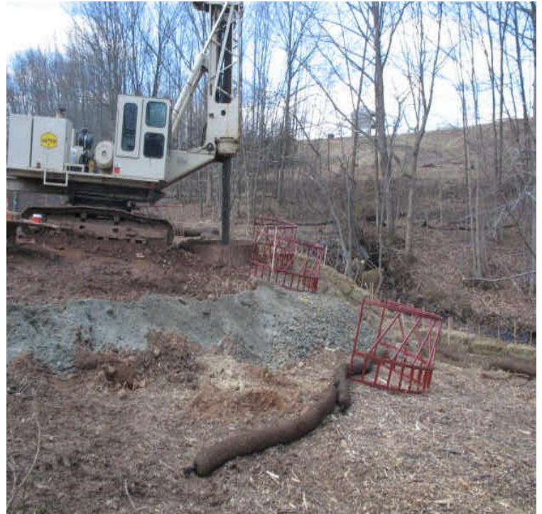
Foundation drilling just north of E. Meriden SS. A slurry pit has been established and will be used as needed. Filter socks are in place around the work. Continue to monitor controls carefully.
