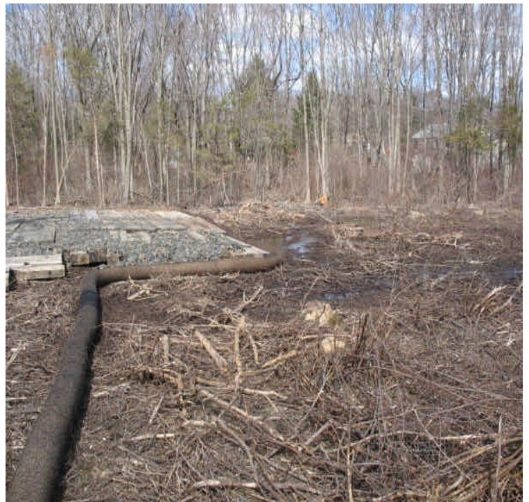
Pad area and controls installed above the stream south of High Hill Road. No run-off noted. Reduce tracking to the timber mat pad to the extent feasible.
