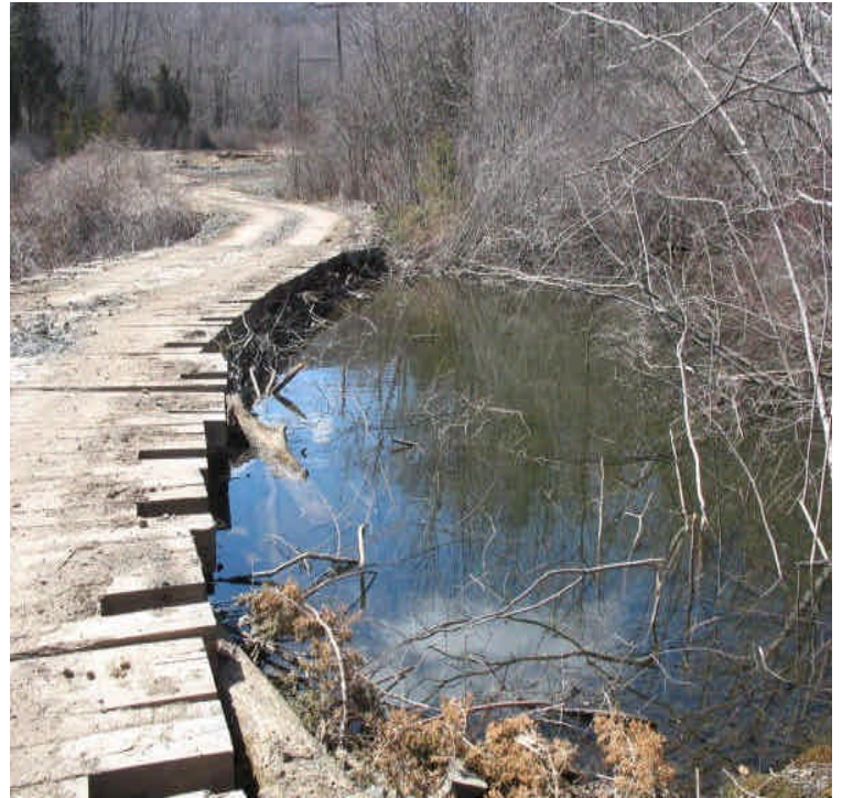
Wetland crossing off Powder Hill Road. Turbidity was not observed within the wetlands at this inspection. Felled trees were removed from the wetlands,
