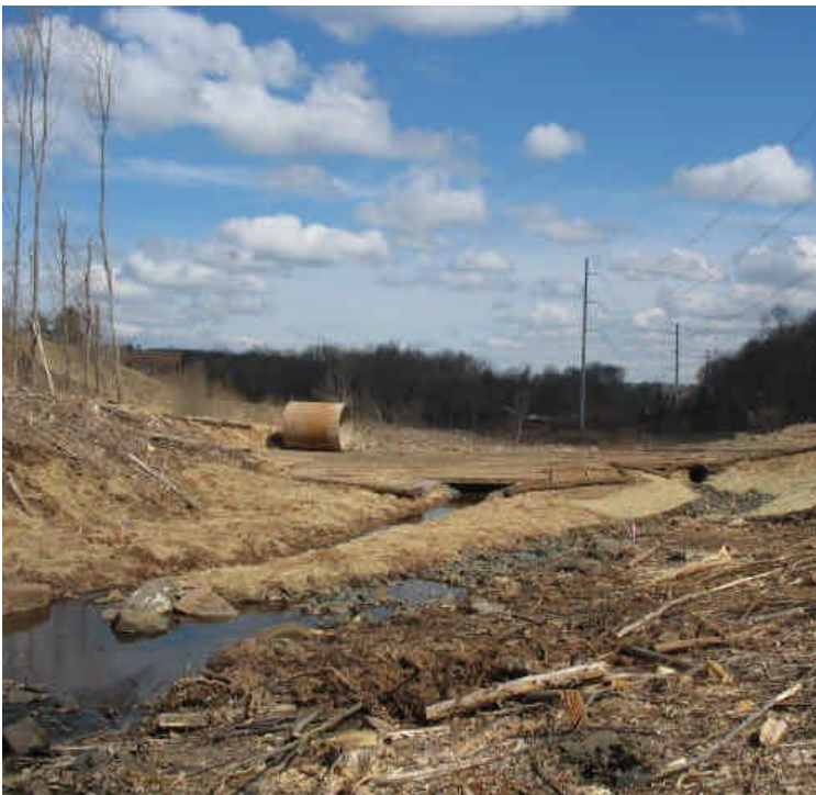
View of the channel banks and adjacent soil temporarily stabilized. in the ROW between E. Meriden SS to Black Pond. Timber mats are in place for workspace and access.
