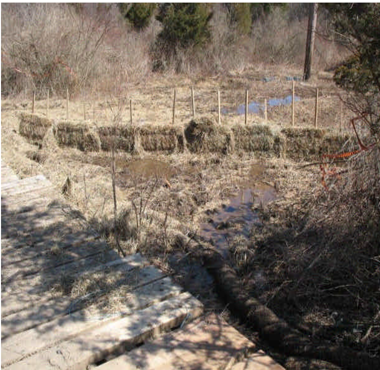
View of newly installed haybales and fiber rolls at the base of the slope off Powder Hill Rd. Sediment is filtered from the run-off before it flows off-site
