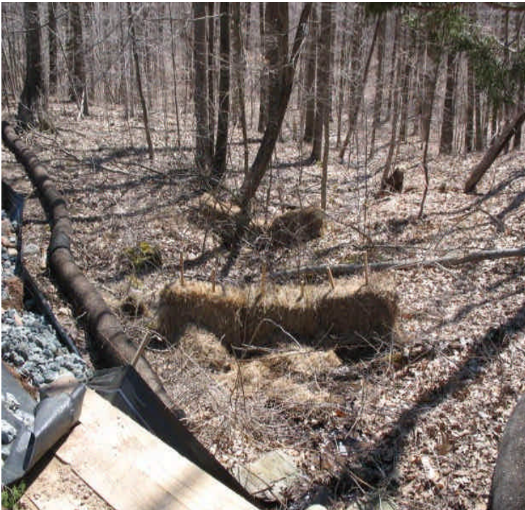
Timber mat wetland crossings have controls, including haybale check dams, installed downgradient off Johnson Lane
