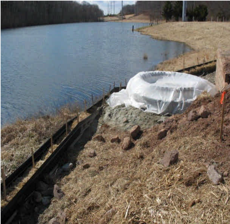
Controls remain in place along the pond north of Beseck SS to E. Meriden SS off Fleming Rd. The foundation at the edge of the pond was installed. Slopes were mulched for temporary stabilization.
