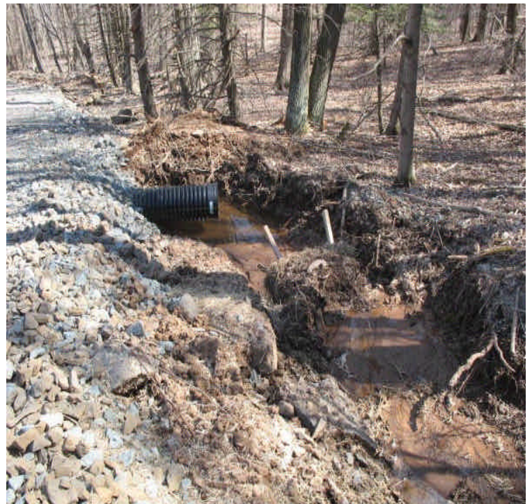
View of the drainage swale with haybale check dams installed along the access road off Powder Hill Rd. Run-off is diverted and filtered prior to leaving the site.
