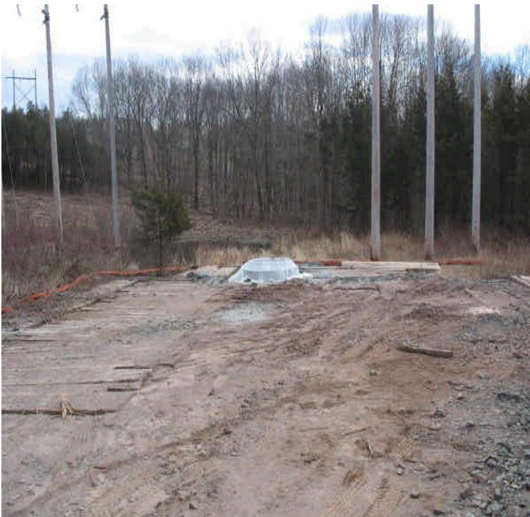
Sediment (likely from snow clearing in past weeks) was noted on and beyond the filter sock at the matted pad near Beseck SS. Sediment in the wetland needs to be carefully removed by hand.
