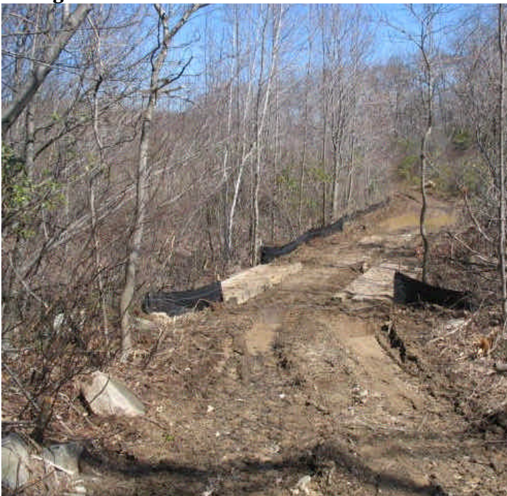
An additional area with controls installed along one of the access roads west of Scovill Rock. The area appears to be well contained.
