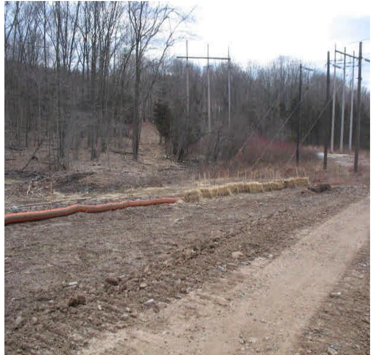
Access road north of Beseck SS has been regraded and stone was added as needed to stabilize the soils and reduce run-off. Haybale and filter sock barriers are in place to slow and contain run-off.
