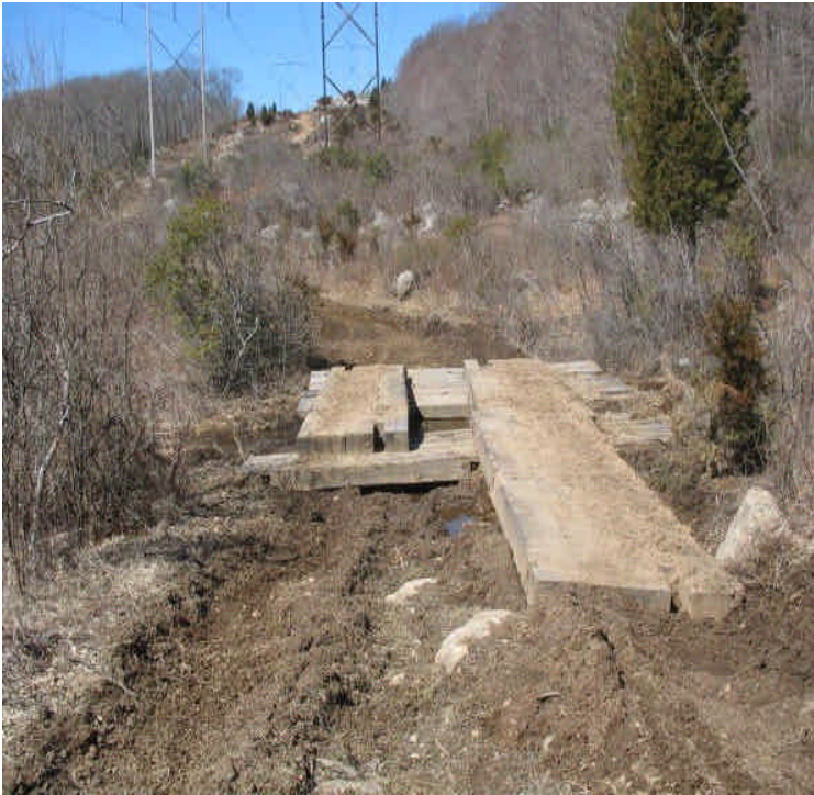
Timber mat crossing within the ROW west of Scovill Rock SS. This was installed for clearing crews access. Crews should work to stabilize soil or place controls after vehicles cause disturbance via tracking
