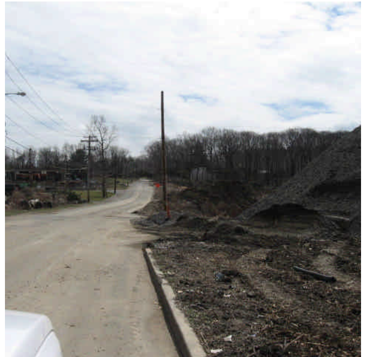
silt saks remain intact in the catch basin. The filter fabric has been pulled over the curb for inlet protection.
