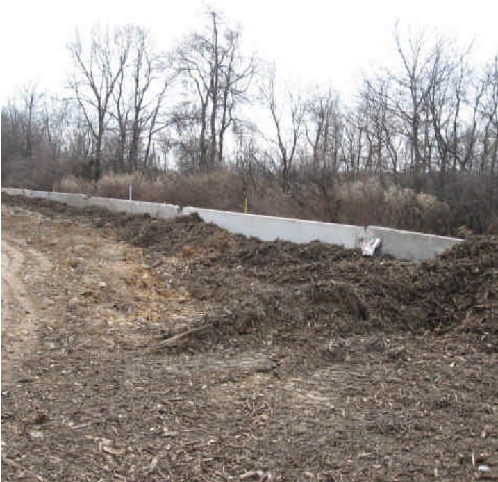
Mulch remains in place at the jersey barriers along the western portion of the site. Minor sediment tracking was noted in Plains Rd. this week but sedimentation is not currently an issue here.
