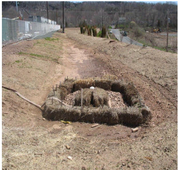
Haybales and controls remain in place at the inlet of the detention basin. Sediment from the stormwater run-off has settled in the basin.
