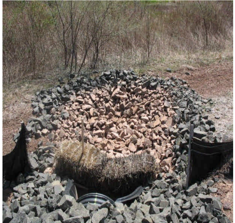
View of the culvert and sediment trap under the access road to the ROW. This control works well for smaller storms but needs reinforcement during the larger rain events.
