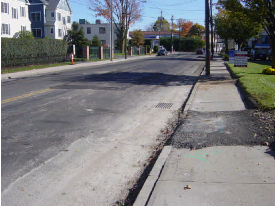
Sediment and granular material has accumulated along the edge of the roadway near sta. #43-45.
