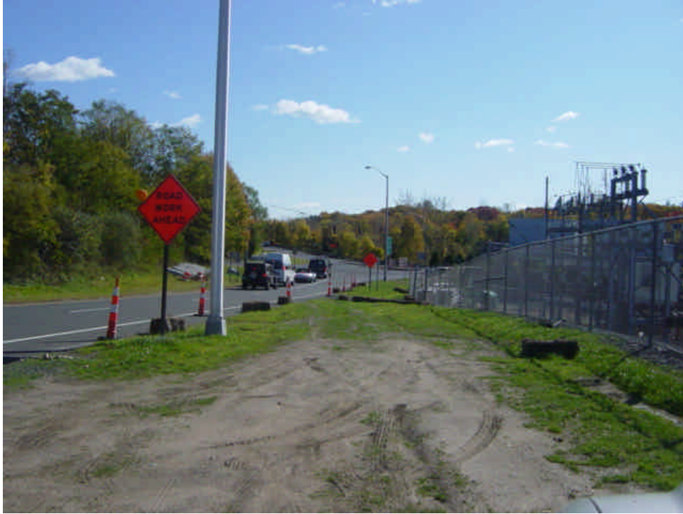
The area outside of the Norwalk substation near sta. #8 has been seeded and the area is beginning to vegetate. The drainage swale has been restored, but sediment has eroded and accumulated in portions of the swale. The receiving catch basin will need to be cleaned.
