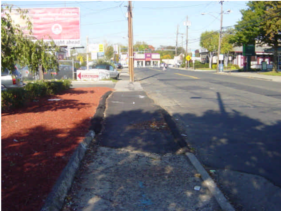
Landscaped area near sta. #31 - 32 has been restored, but curb and sidewalk restoration is still required.
