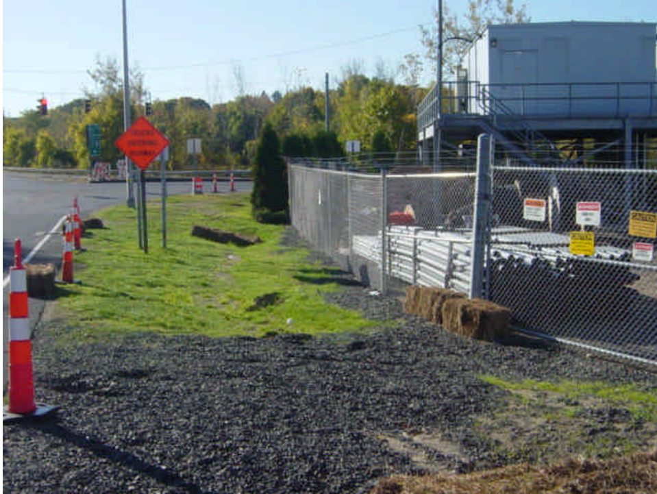
The area outside of the Norwalk substation near sta. #8 has been seeded and the area is beginning to vegetate. The drainage swale has been restored, but sediment has eroded and accumulated in portions of the swale. The receiving catch basin will need to be cleaned.
