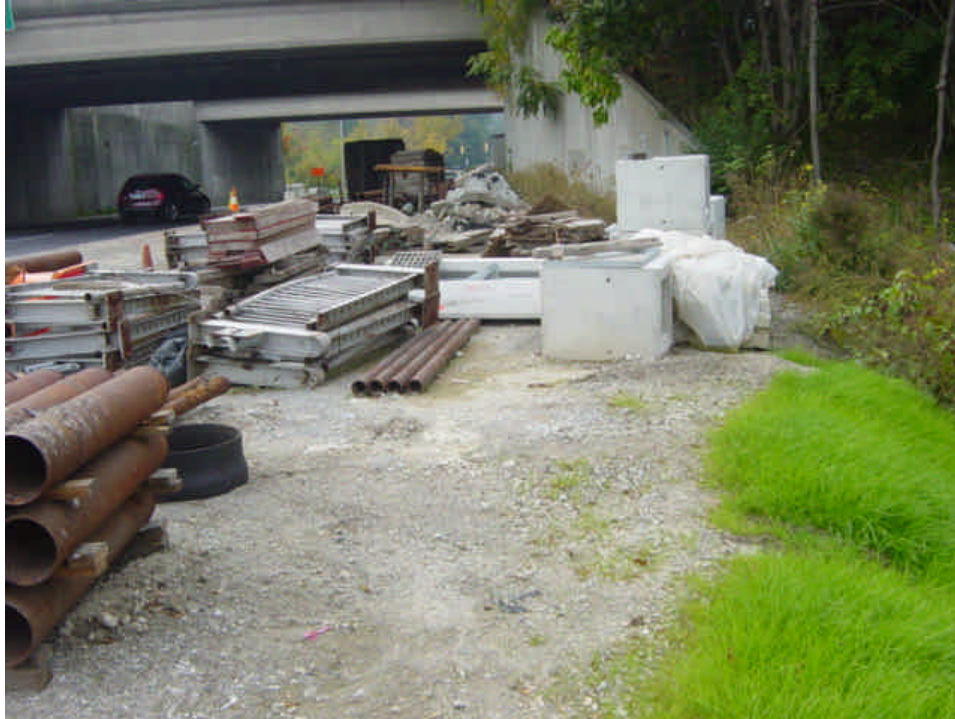
The slope at sta. #14-18 has been re-graded and is stabilized, except for a portion near the road where exposed soil remains. Material for the adjacent bridge project is also being staged in this area.
