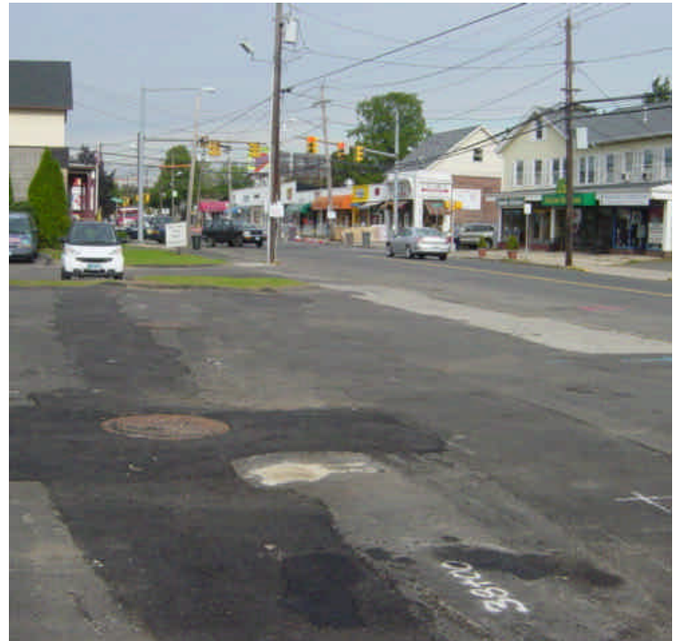
Tie-in work has been completed near sta. #38 and the area has been temporarily paved.
