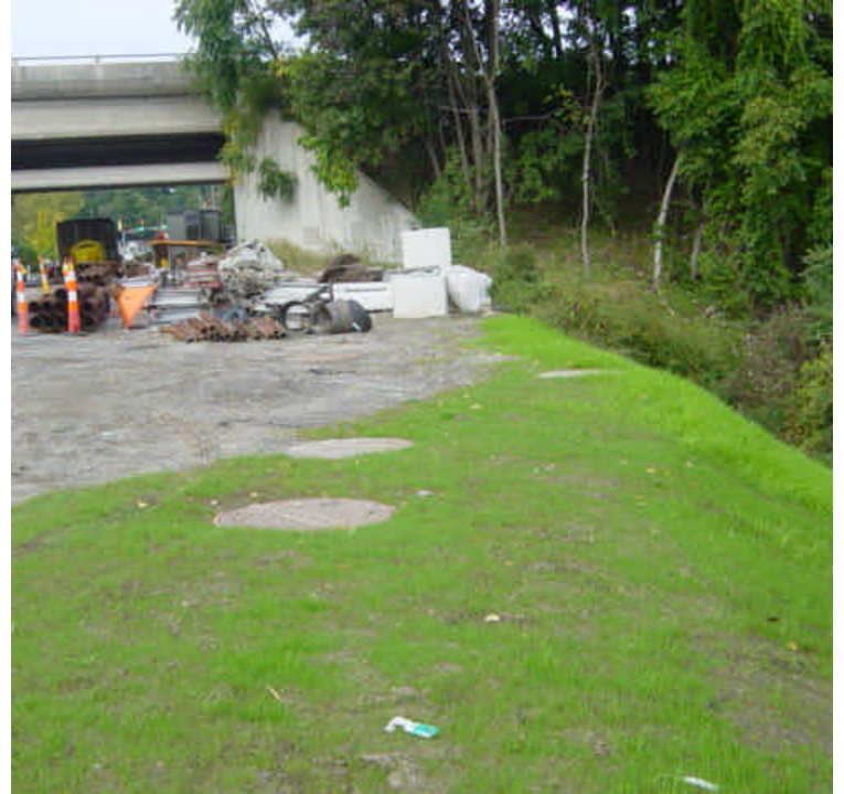
The slope at sta. #14-18 has been re-graded and is approximately 65% vegetated. Silt fence and hay bale barrier remains along the graded slope. Construction materials noted here are not related to the M/N project.
