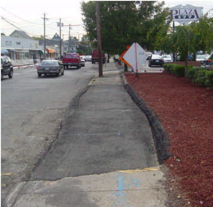
The median area near sta. #31+50 has been restored. Additional restoration to the curb and sidewalk is still required.
