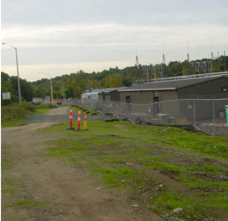
The area outside of the Norwalk substation near sta. #0-4 has been seeded and the area is beginning to vegetate. The drainage swale has been restored however, heavy rain has caused portions of the swale to fill in with sediment.
