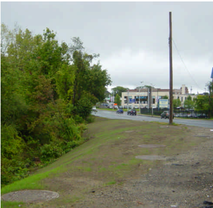
The sloped area near sta. #14-18 has been restored and is beginning to vegetate. Mulch may still be needed until grass cover can establish.
