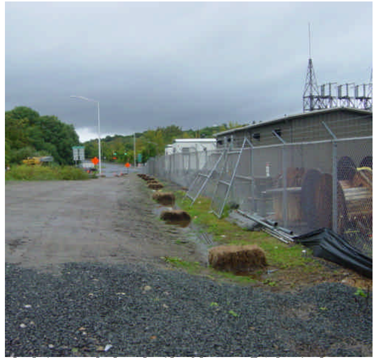
The drainage swale along the side of the Norwalk Substation has been restored. Haybale check dams are in place. However, heavy rains caused portions of the swale to fill with sediment. Exposed soil needs mulch and seed.
