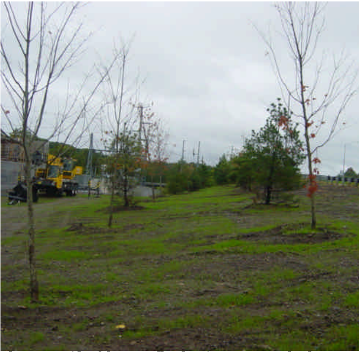
The area outside of the Norwalk substation near sta. #0 has been (including hydroseed) and the area is beginning to vegetate.
