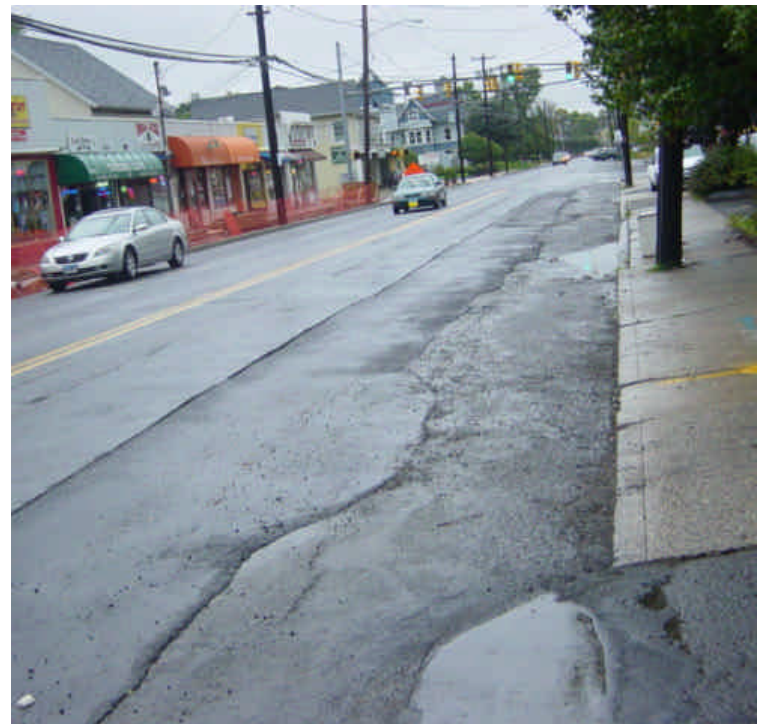
Trenching is complete along Main Street. A minor amount of cold mix remains along the edge of the roadway. Sweep roadways when feasible.
