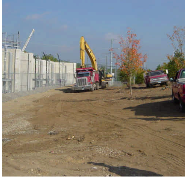
Pre-cast concrete retaining wall has been restored outside of the Norwalk substation near sta. #0 and the area has been backfilled. Some trees and landscaping has also been restored. Exposed soil needs mulch and seed.
