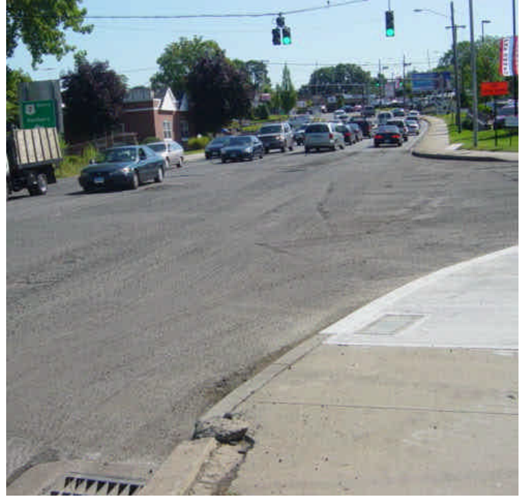
Pavement has been milled near sta. #19-21 and is ready to be paved.
