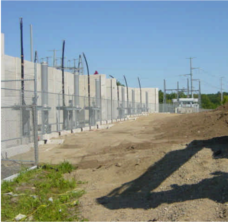
Pre-cast concrete retaining wall has been restored outside of the Norwalk substation near sta. #0.
