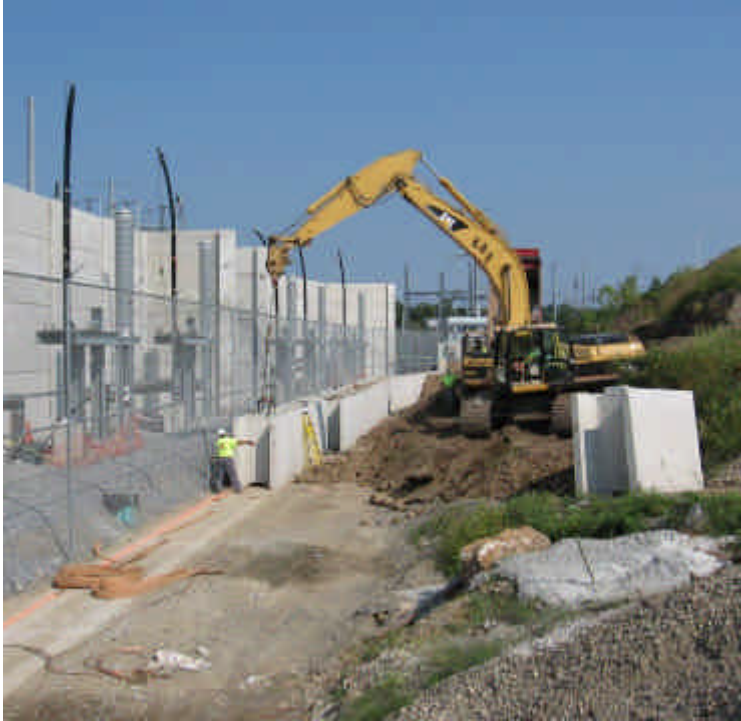
Pre-cast concrete retaining wall was being re-set outside of the Norwalk substation near sta. #0.
