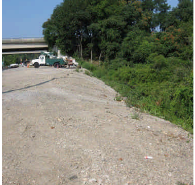
Evidence of multiple concrete washouts remain along the slope near sta. #14-16. There is no active work in this area and the washouts are likely not project related. However, the area remains exposed for several months and needs temporary or permanent stabilization.
