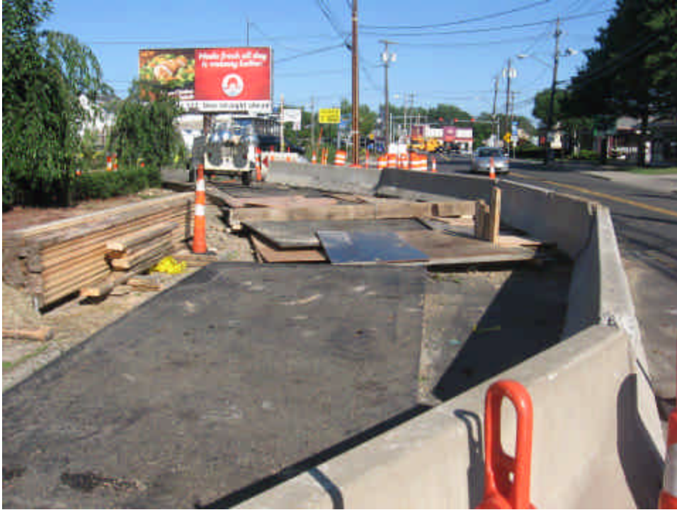
Steel plates were in place over the trench near sta. #32-33. Concrete barriers were also in place around the work area.
