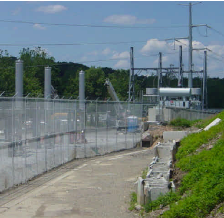
Tie-in work has been completed at the Norwalk substation. The pre-cast concrete wall needs to be restored.
