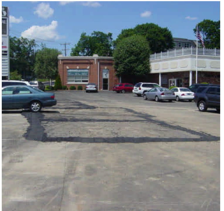
Trenching continues near sta. #52-53. Steel plates were covering the trench at the time of the inspection. A minor amount of granular material was observed along the edge of the roadway/ parking lot. Sweep as needed.
