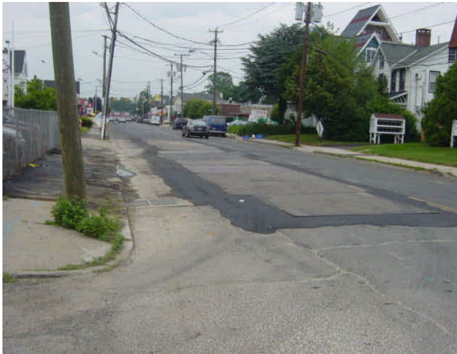
Trenching continues near sta. #40-41. Steel plates were covering the trench at the time of the inspection. A minor amount of granular material was observed along the edge of the roadway adjacent to the catch basin. Sweep as needed and clean the catch basin.
