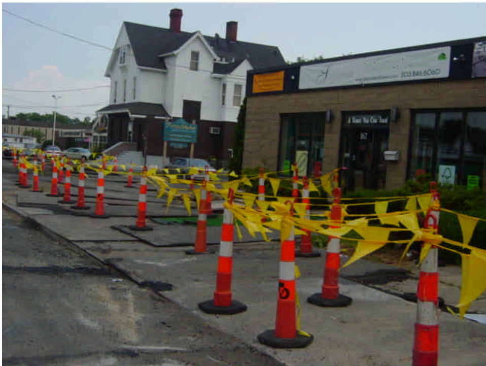
Steel plates remain in the parking lot area over the trench near sta. #36-38.
