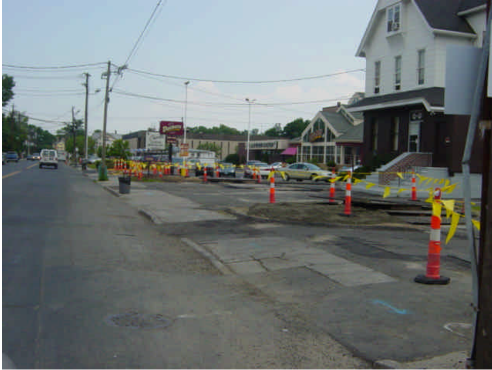
Trenching continues near sta. #36-38. Steel plates were covering the trench at the time of the inspection. Sweep roadway as needed.
