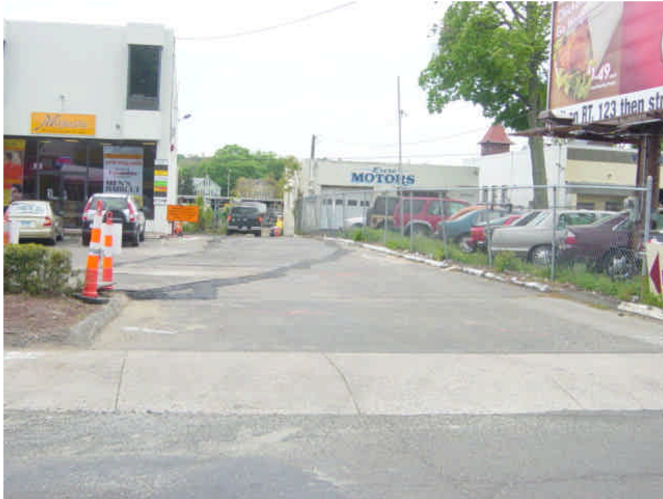
Trenching continues between sta. #28-30. Steel plates were covering the trench at the time of the inspection.
