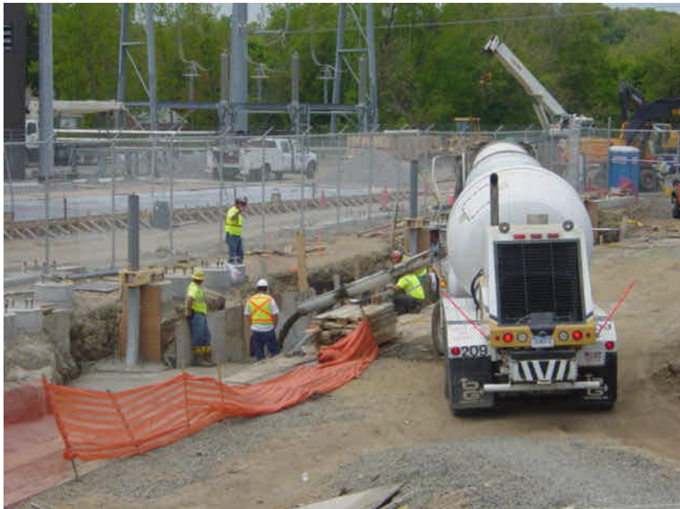
Conduit has been installed to the bases of the previously placed foundations and the Trench between sta. #0-2 was being backfilled.
