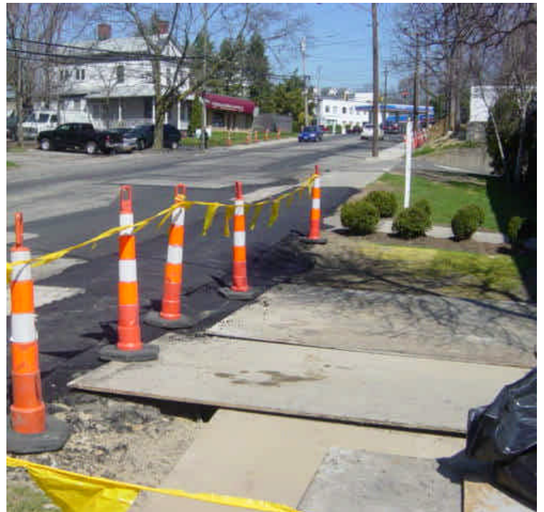
Trenching continues near sta. #50-51. Steel plates are in place along the roadway and adjacent parking lot.
