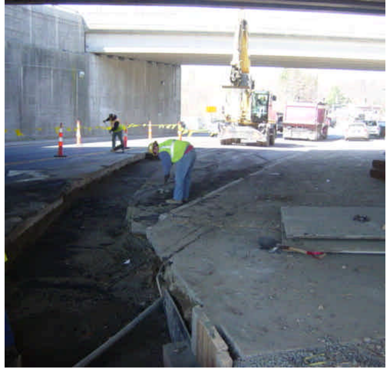
Backfilling continues between sta. #13-14. Crews were sweeping the roadway to reduce the potential for tracking.
