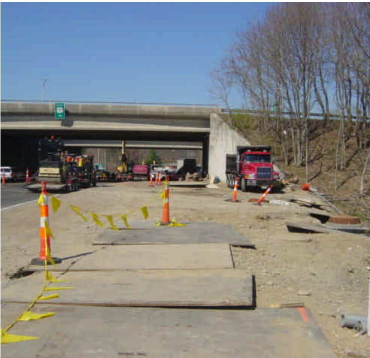
Steel plates are in place near sta. #15 and handholes are being installed. Silt fence remains in place along the toe of the slope, but sediment is beginning to accumulate here.
