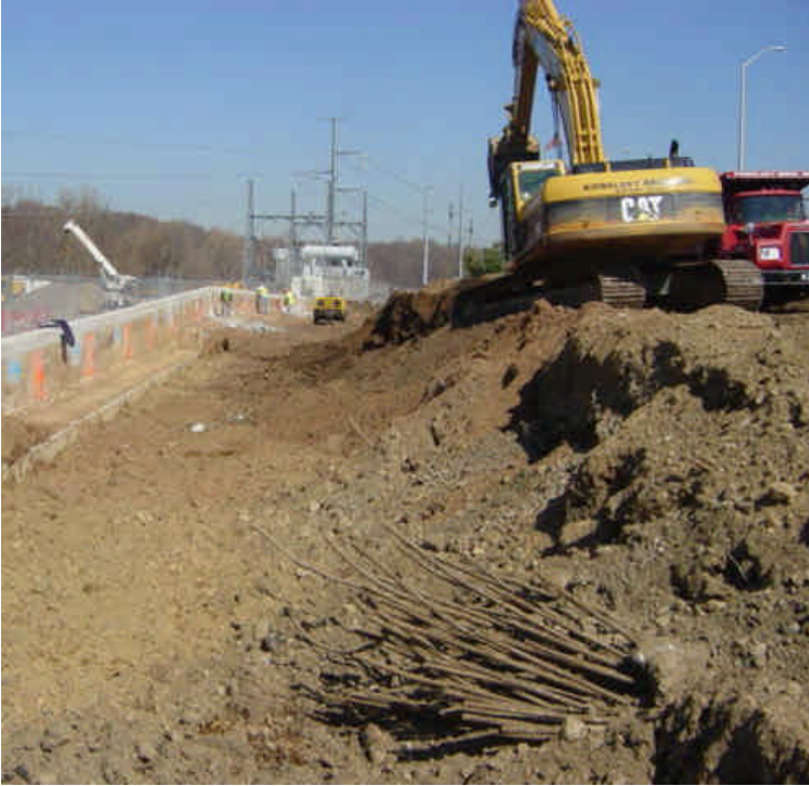
Earthwork is being performed near sta. #1-3 in preparation for final trenching to tie-in to the Norwalk Substation.
