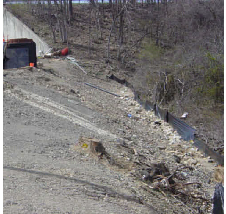
Silt fence remains in place along the slope between sta. #15-18. Sediment and debris are beginning to accumulate along the fence.
