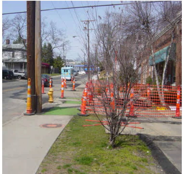
Trenching continues near sta. #50-51. Steel plates are in place in the roadway and adjacent parking lot.
