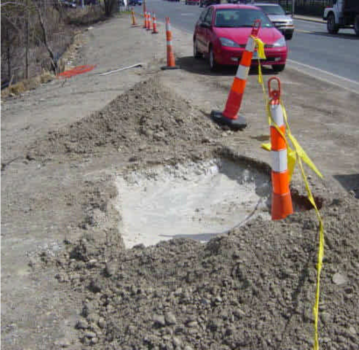
A concrete washout area was observed near sta. #16. Attempts were made to contain the area but additional controls are needed. The dirt berms should be built up if the area will be used further.
