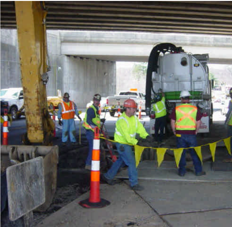
Trenching activities continue near sta. #13-14. The trench was being properly dewatered using a vac truck.
