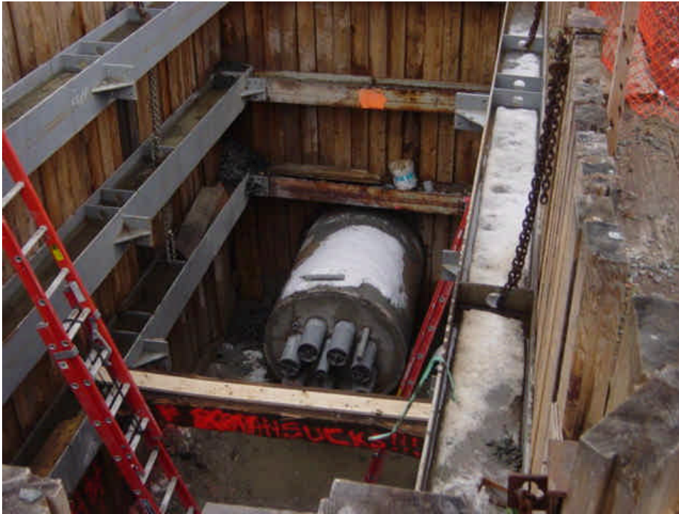
View of the conduit and casing at the jack and bore pit near station #25, where the project crosses a railroad bed.
