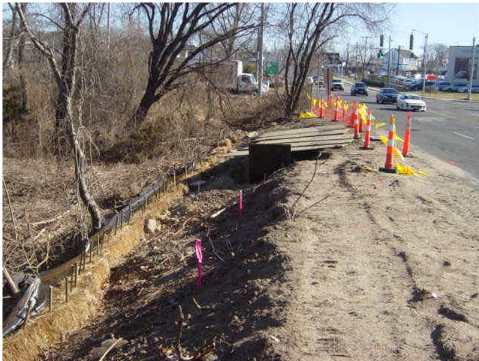
Another view of the hay bale and silt fence barrier in place along the slope between sta. #15 to 18. Controls are in good shape. No active work was occurring at the time of this week's inspection
