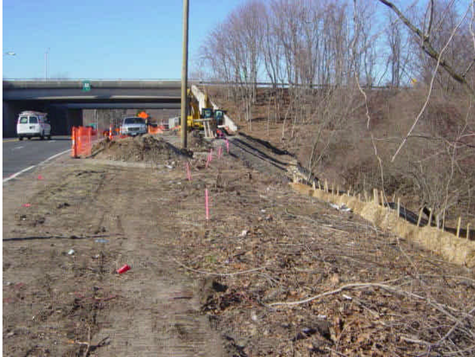
The hay bale and silt fence barrier has been extended along the slope between sta. #15 to 18. Some small stockpiles were noted in the work area.
