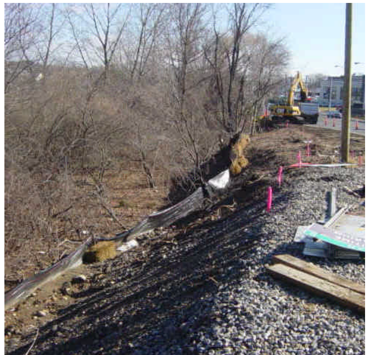
The hay bale and silt fence barrier has been extended along the slope between sta. #15 to 18. Trenching continues near sta. #18. A hay bale has also been placed between the break in the silt fence near sta. #15.
