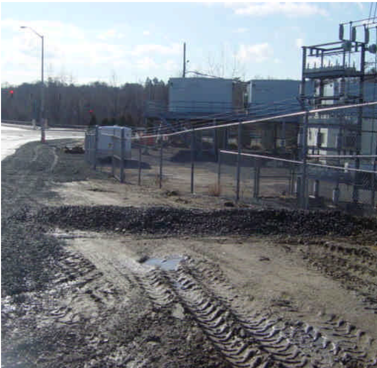
A stone berm has been placed along the shoulder of the Rte. 7 off-ramp near sta. #8 to direct run-off away from the entrance to the adjacent substation. Ensure that this solution does not result in problems to the roadway instead.
