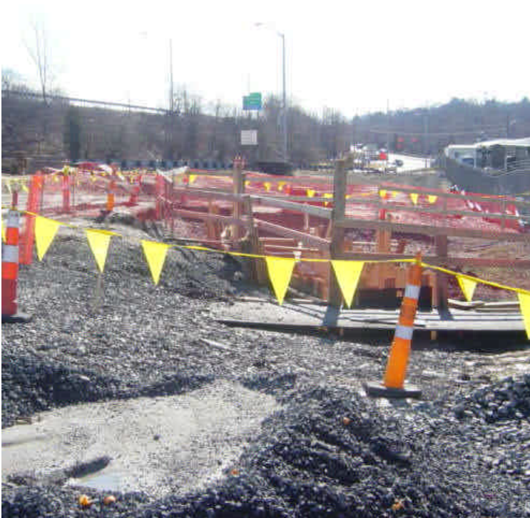
Trench between sta. #3 to 4 has been partially backfilled but remains open. A properly contained concrete washout area was established near the trench.
