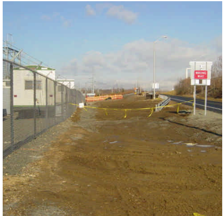
Drainage swale has been partially restored between sta. #4+50 to 6+50. Crushed stone has been placed along the swale. Surrounding areas have been temporarily backfilled with process material and graded. When conditions allow, evaluate whether landscaping and vegetation should be restored.
