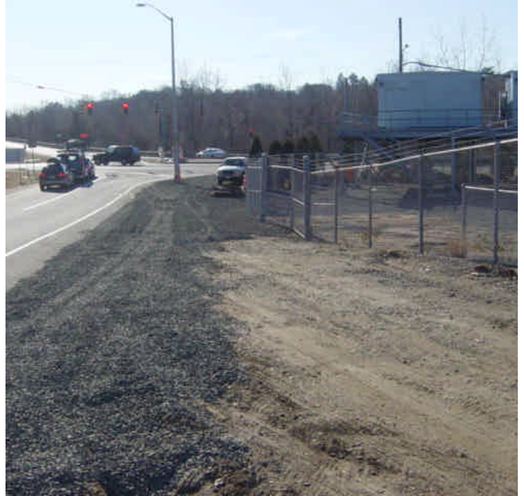
Crushed stone has been placed over areas of exposed soil along the shoulder of the Route 7 off ramp near sta. #9. Additional erosion control measures may still be required to direct surface runoff away from the substation gate, where sedimentation has previously occurred. Permanent drainage restoration will also be needed at the conclusion of the work
