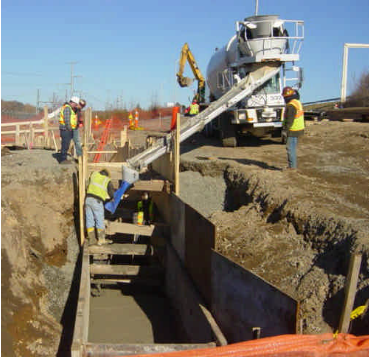
Trenching and backfilling work continue near sta. #4 along the Norwalk substation fence and the Rt. 7 off-ramp.
