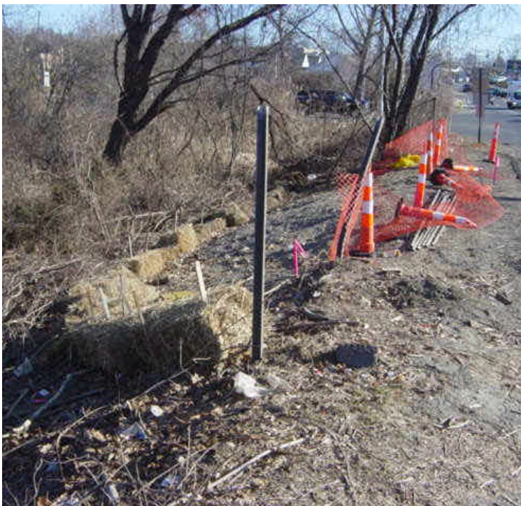
The haybale barrier near sta. #18 has been re-established and the haybales are properly staked to the ground.
