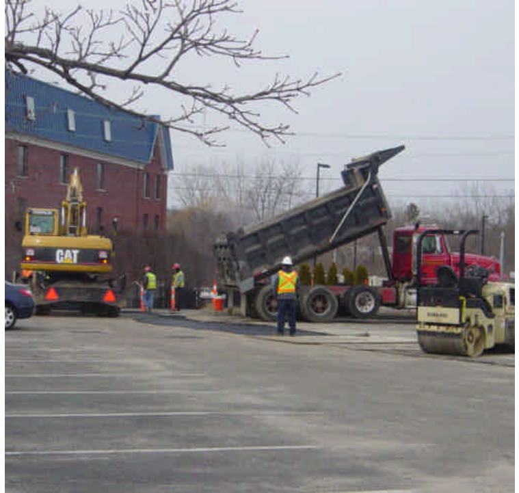
Trenching activities have been completed near sta. #23-24 and crews are re-paving the area.
