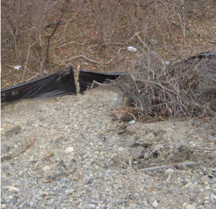
Silt fence has been repaired near sta. #15-16 but there is a small break in the fence, where a gully has formed. Sediment is eroding in this location and is beginning to migrate beyond the silt fence barrier.
