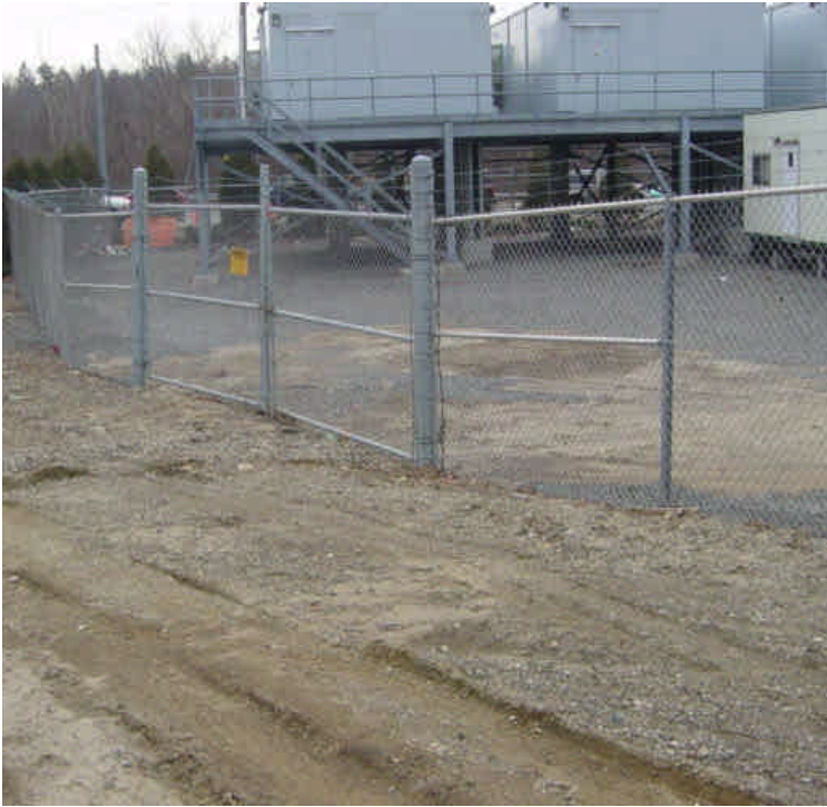
Exposed soil along the Route 7 off ramp near sta. #9 has eroded and sediment has migrated into the adjacent substation. Contractors stated that they placed additional stone here following the inspection.
