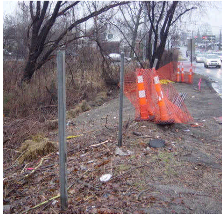
Haybales down gradient of the slope at station #18 have been moved, no longer forming a continuous barrier. Haybales need to be reset and staked to form a continuous barrier. Exposed soil should be temporarily stabilized for the winter.
