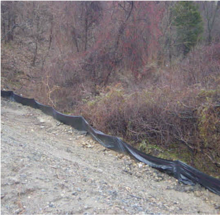
Silt fence was repaired appropriately at station #15-16. Exposed soil should be temporarily stabilized for the winter.
