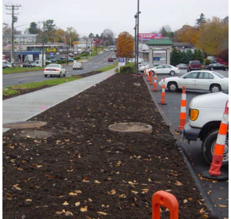
Area near sta. #129-130 has been partially restored. Topsoil has been spread but remains exposed and needs to be stabilized/winterized with mulch.
