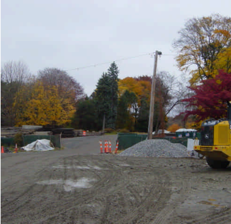
No tracking or dust issues were observed at the Sherwood Island lay-down yard.
