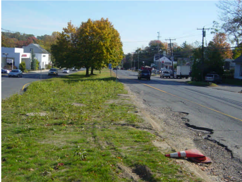
The area near sta. #316-318 has vegetated with weedy growth. Ruts and eroded gullies were observed in a few locations. Bituminous curbing and edge of pavement still need to be restored.
