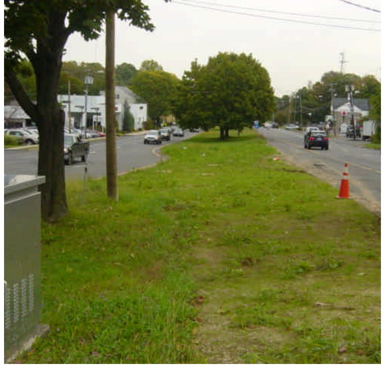
The area near sta. #316-318 has vegetated with weedy growth. Bituminous curbing still needs to be restored.
