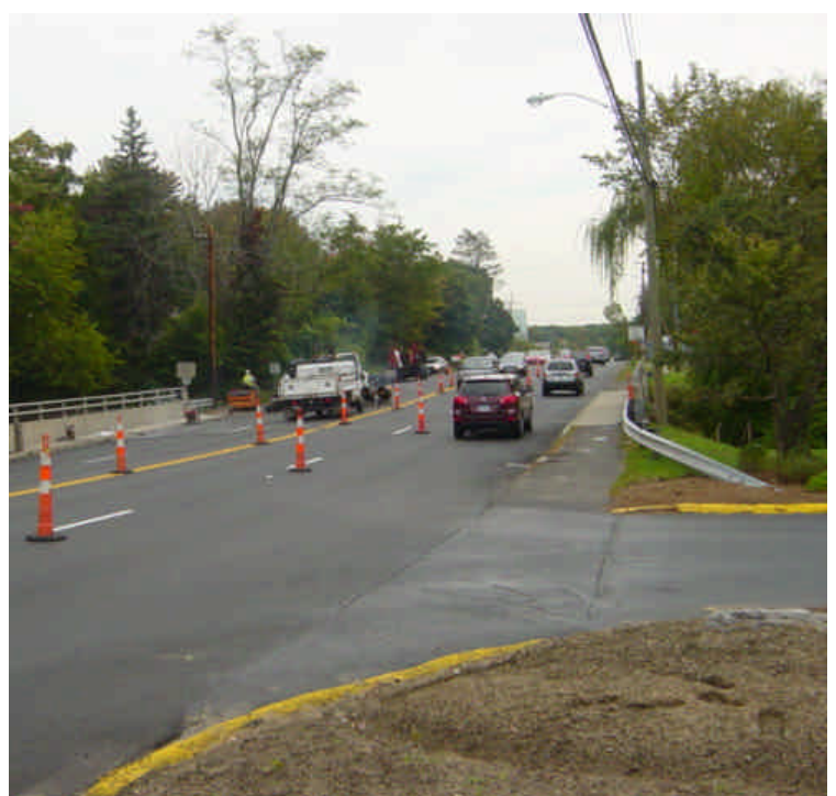
Asphalt road work was observed near sta. #435 at the Sasco Creek bridge crossing.
