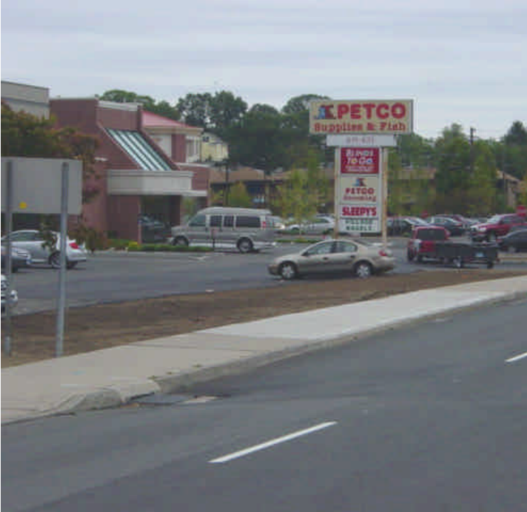
Topsoil has been spread in the area near sta. #146 and the area is partially restored. Continue to mulch/stabilize exposed soils.
