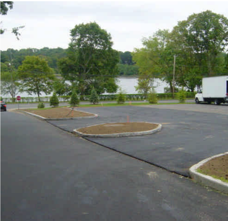
Parking lot near sta. #234 has been repaved and the island areas have been seeded. Mulch should be added to further stabilize.
