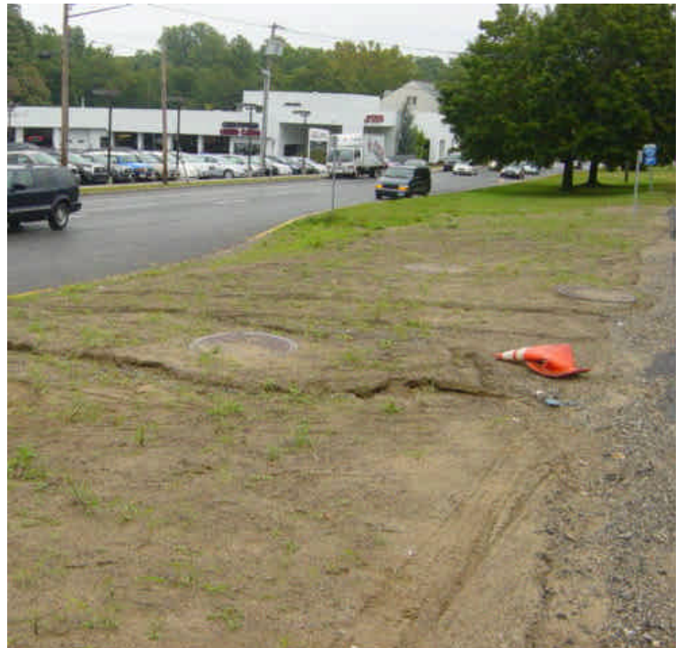
The area near sta. #316-318 was previously graded and seeded. However, heavy rain has caused portions of the exposed soil to erode and gullies were present. The area will need to be repaired and mulch should be applied.
