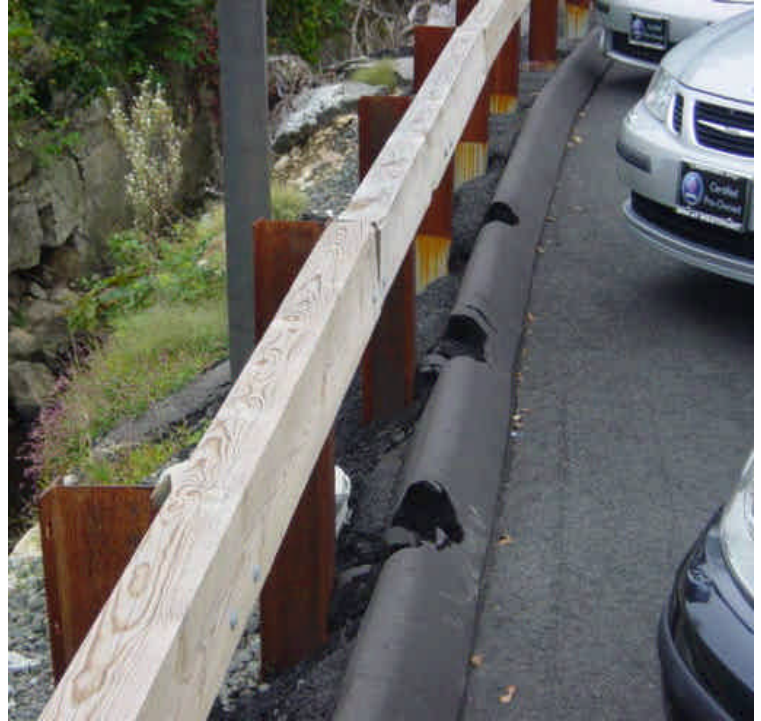
Bituminous curb was previously restored near sta. #217, but several areas have been damaged.
