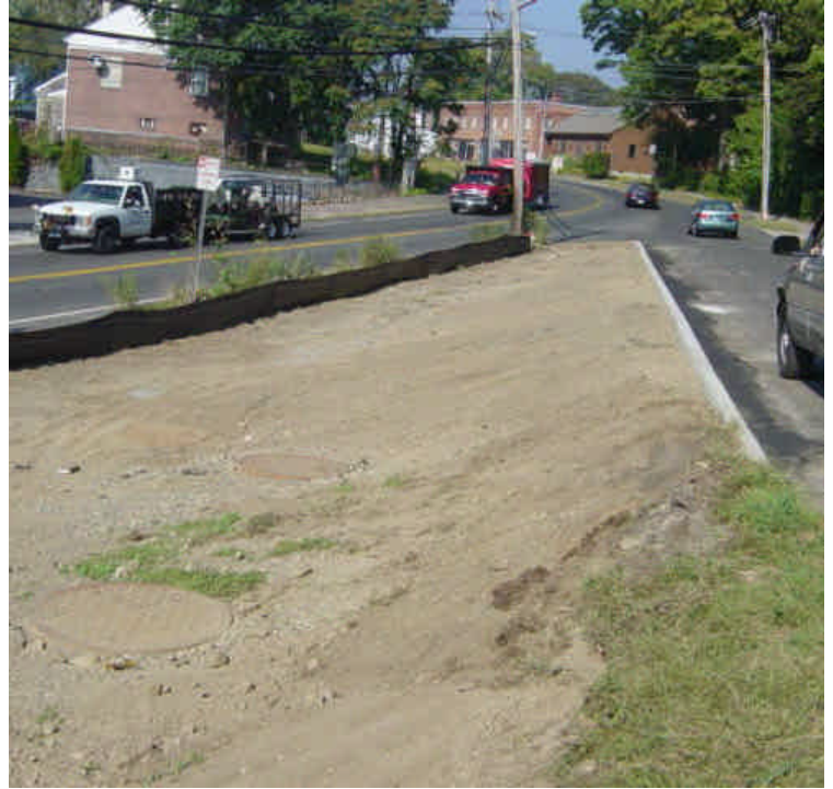
Stone curb has been reset near sta. #81 and topsoil has been spread. Provide stabilization for the exposed soil as soon as feasible.
