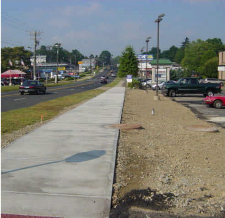
Topsoil has been spread in the area near sta. #130. Light poles and sidewalk have also been restored. Stabilize the exposed soil with mulch and seed as soon as possible.
