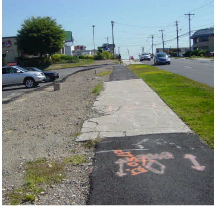
The area near sta. #130 remains backfilled with process material. Final restoration is needed in this area.
