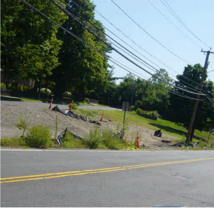
Temporary curbing remains along Westport Ave. near sta. #81 (vault #5) but is beginning to deteriorate. Silt fence needs repair.
