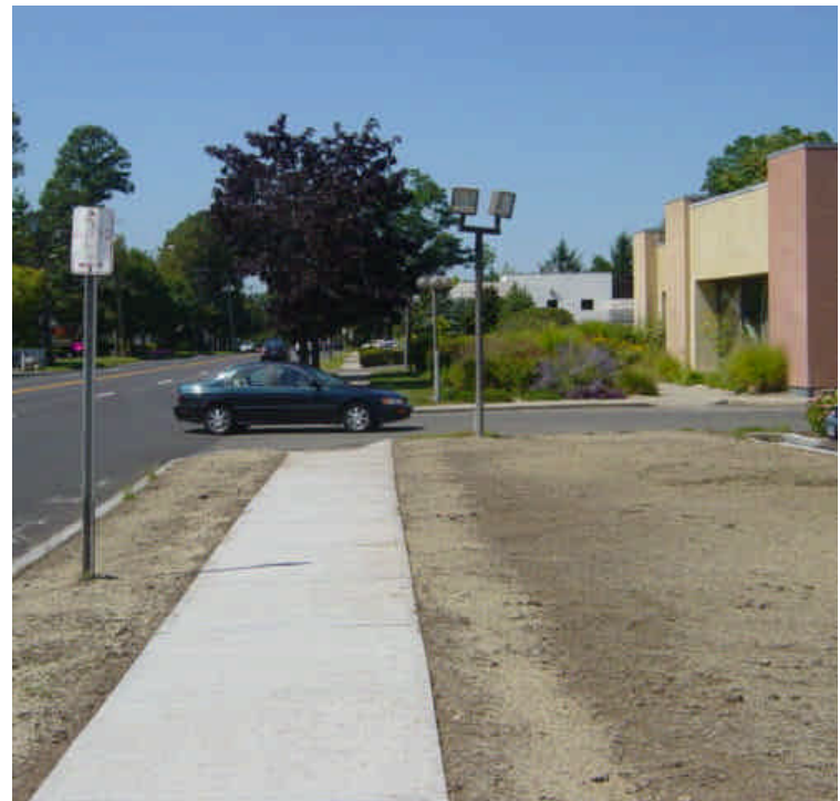
Topsoil has been spread near sta. #381-383. The exposed soil needs to be seeded and stabilized. Efforts are underway.
