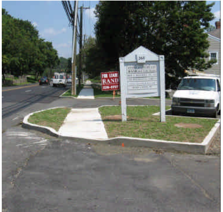
A minor amount of debris/sediment was observed along the edge of the curb near vault #12, where restorations efforts are underway.
