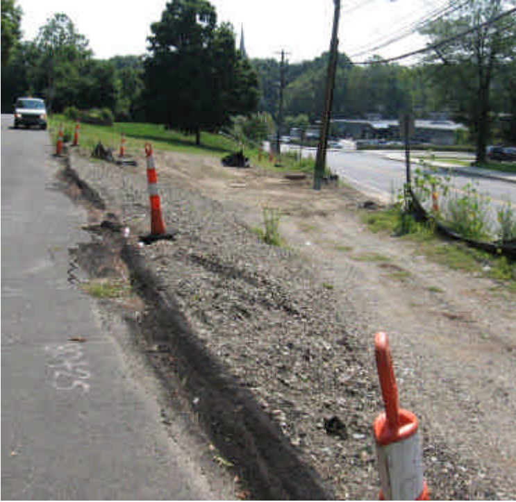
Temporary curbing remains along Westport Ave. near sta. #81 (vault #5) but is beginning to deteriorate. Area has been backfilled with process material but remains exposed. Work towards final stabilization/surfacing in the area.
