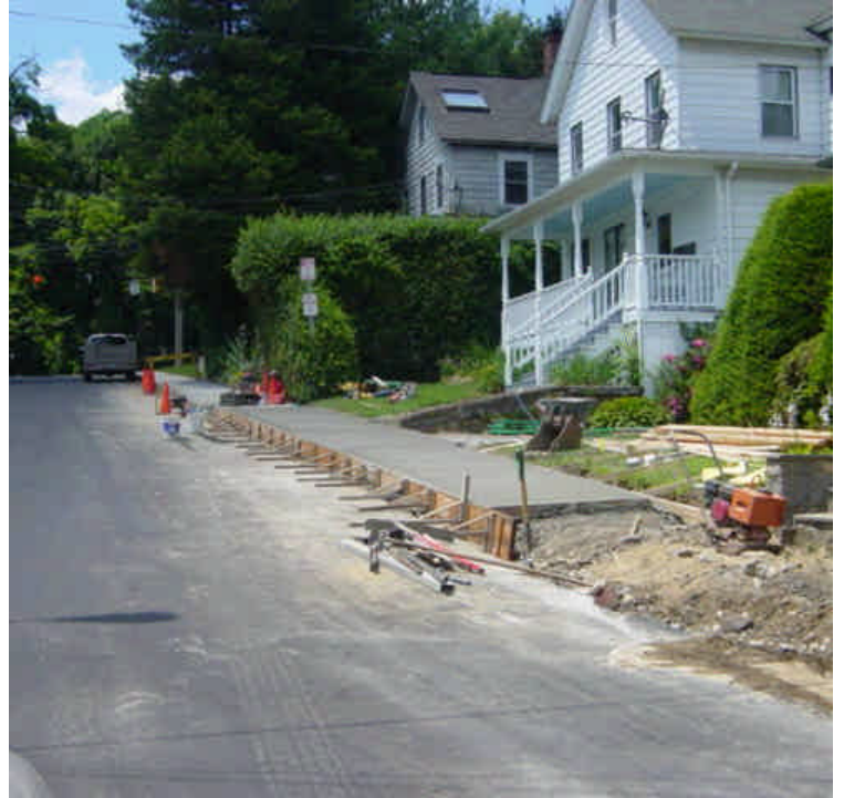
Sidewalk restoration was observed near sta. #230. This work was not project related.
