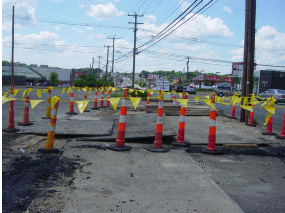
Steel plates remain in the parking lot near sta. #162-164. A minor amount of loose cold mix and sediment has accumulated along the edge of the plates.
