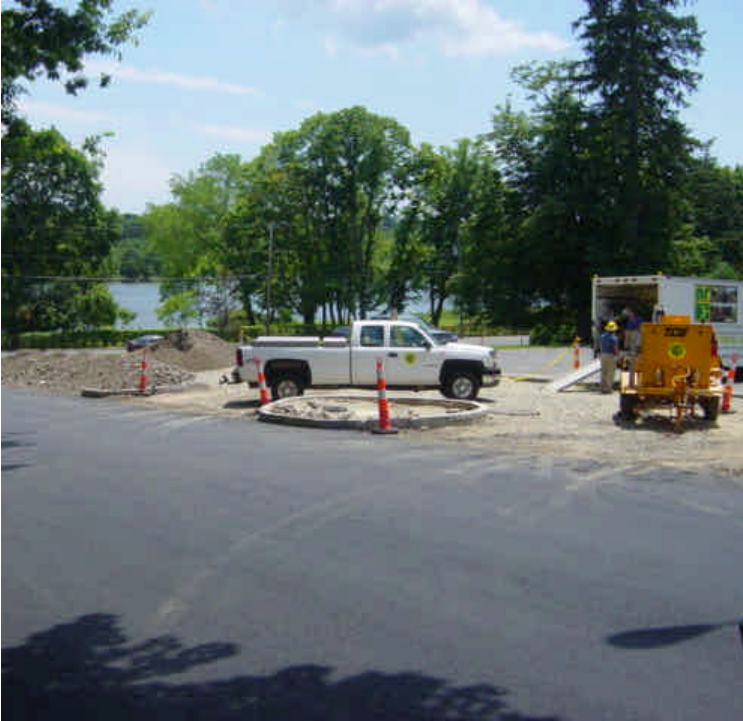
On the west side of the Saugatuck River, the staging area is still waiting to be paved. Stone curbing has been set and soil has been stockpiled in these areas. Minor tracking was observed on Lincoln St. New River Electric was on-site.
