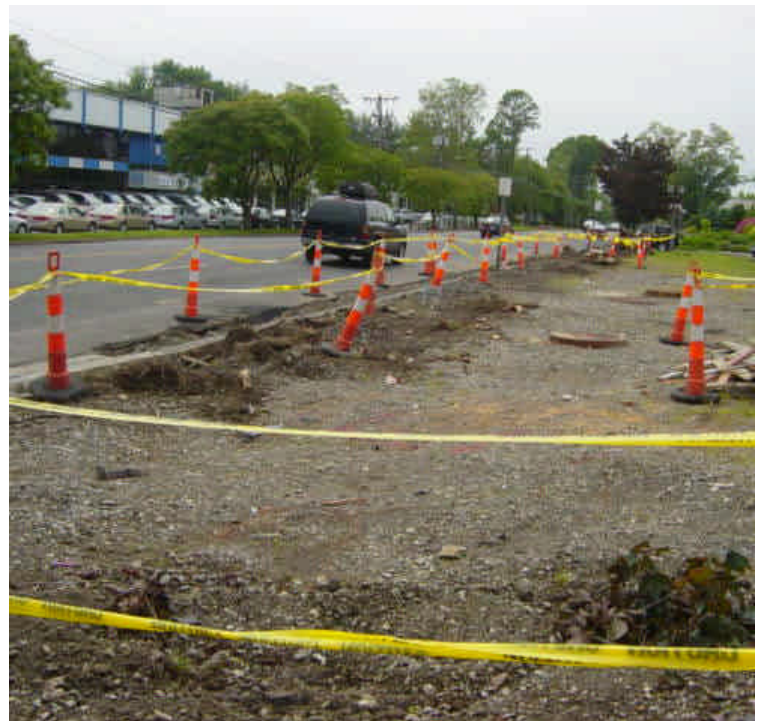
Restoration work is underway near sta. #382. Concrete formwork is in place for new sections of curbing.
