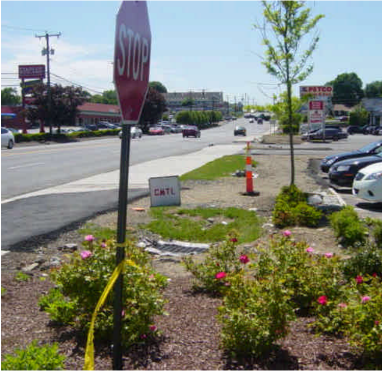
Work appears to be complete near sta. #148. The sidewalk has been temporarily restored with bituminous pavement. Restore grass cover over the trench when feasible.
