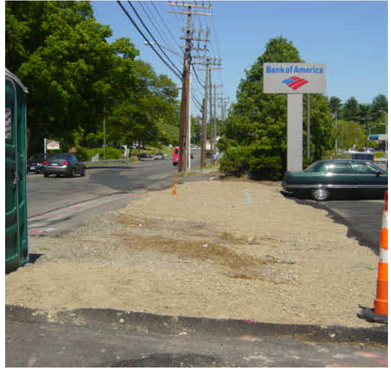
Work continues near sta. #163-164. Steel plates remain over the trench in the parking lot area.
