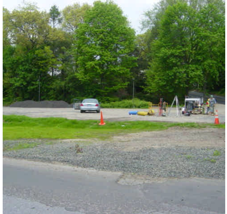
The staging area on the east side of the Saugatuck River has been restored. Electrical contractors were on site proofing the lines.
