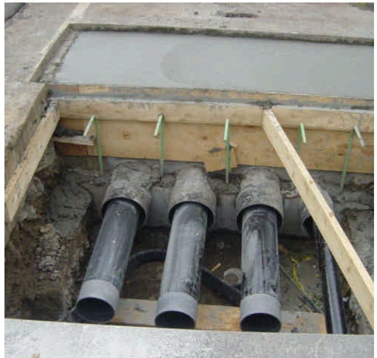
Work continues on the bridge over Sasco Creek continues near near sta. #434 as conduit sleeves were being installed under the bridge deck.
