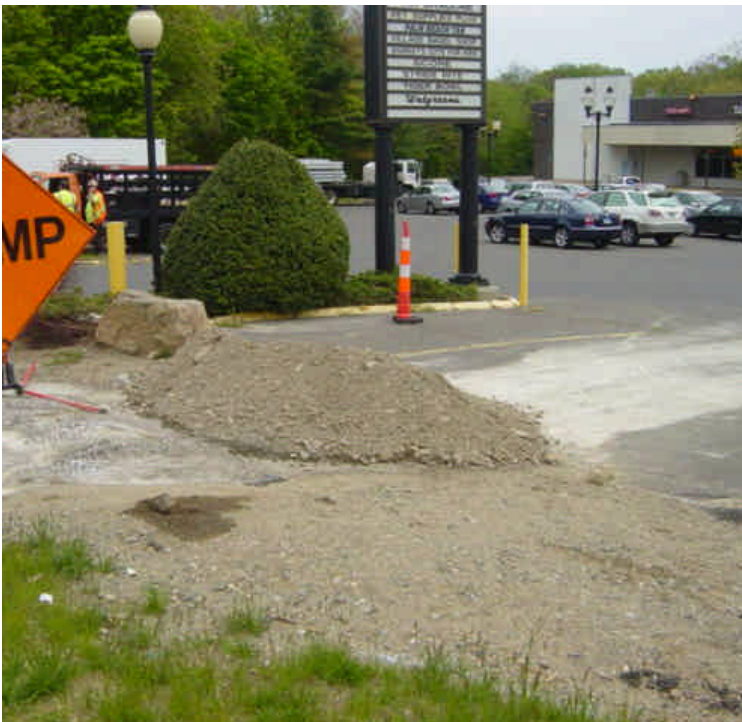
A small soil stockpile was observed near sta. #433+65. The material appeared to have migrated into the parking lot. Use controls or temporarily stabilize the soil.
