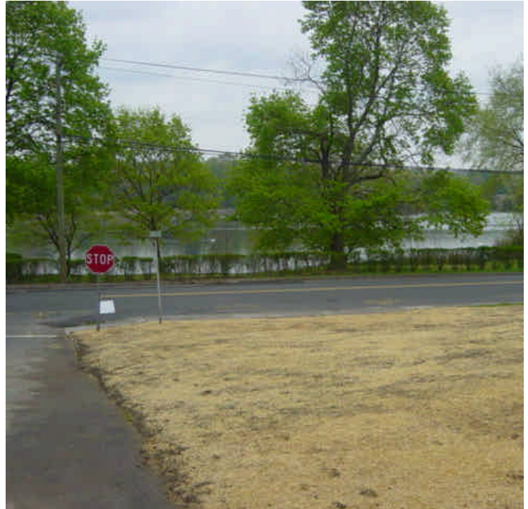
Area of exposed soil near sta. #231 was previously seeded and grass cover was beginning to establish.
