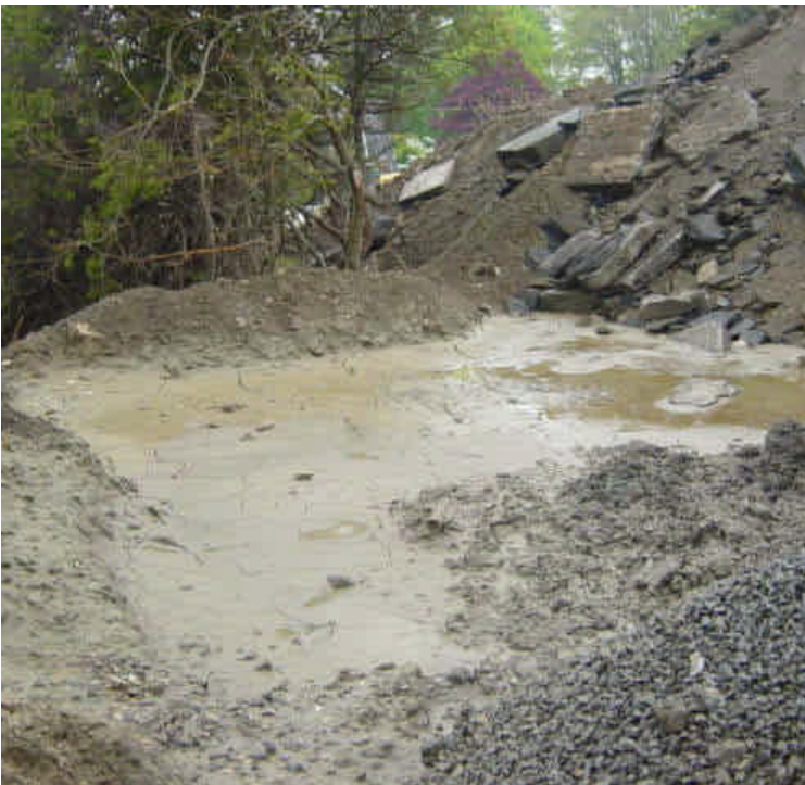
Frac tank washout water has been mixed with the material stockpile in the Sherwood Island yard to bind the material for disposal.
