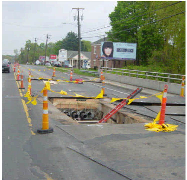
Work continues on both sides of the bridge over Sasco creek near sta. #435 in preparation for hanging the conduit from the bridge deck.
