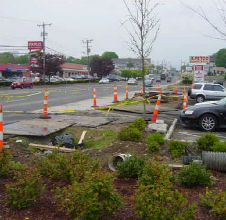
Trenching and vault tie-in work continues near sta. #148-149. The area was covered with steel plates at the time of the inspection.
