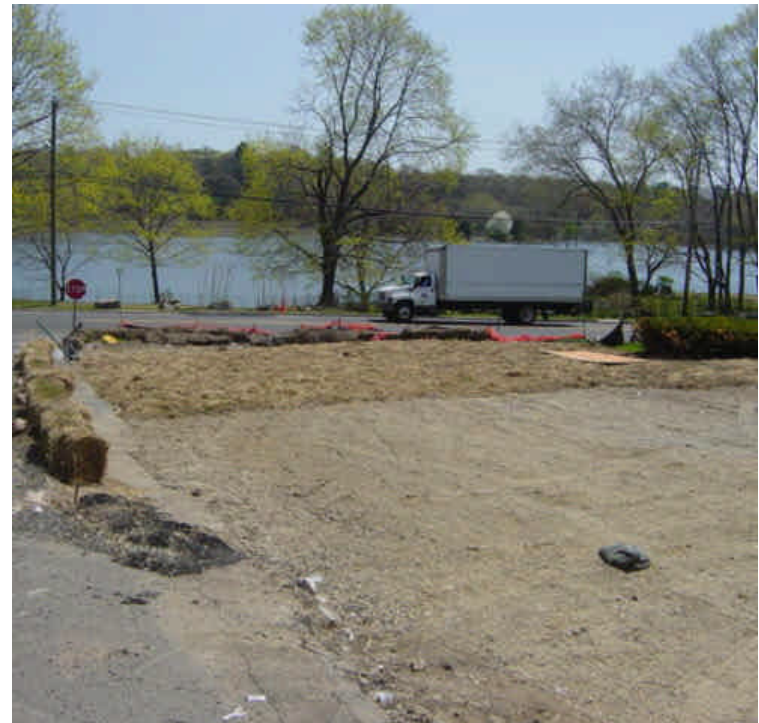
The area near sta. #231-234 has been prepared for paving for several weeks. Seed and mulch were previously spread over the portion of exposed soil that is not slated for paving.
