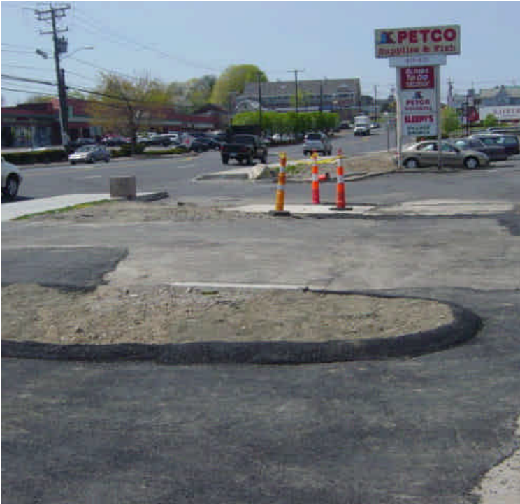
Trenching continues near sta. #147. Plywood is being used to temporarily cover the catch basin during construction activities. However, evaluate whether this is adequate for control.
