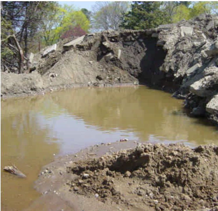
Frac tank washout water has been mixed with the material stockpile in the Sherwood Island yard to bind the material for disposal.
