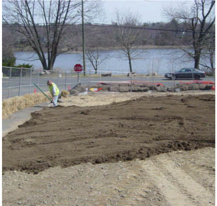
Tie-in work has been completed near sta. #234. The area has been backfilled and topsoil and seed were being applied.
