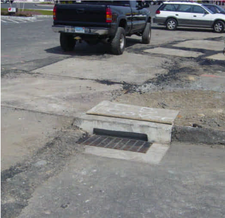
Trenching continues near sta. #147. Plywood is being used to temporarily cover the catch basin during construction activities.
