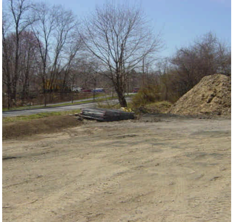
Tie-in work is complete near sta. #251. The staging area has been partially restored. Wood chips and chain link fencing remain stockpiled in the staging area. A dirt berm was recently re-graded.
