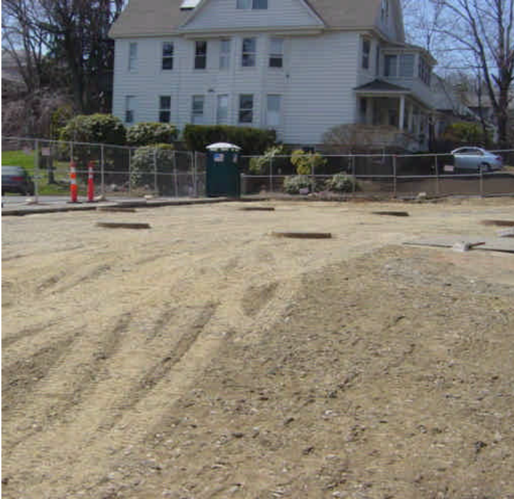
Tie-in work has been completed near sta. #234. The area has been backfilled and this portion is ready to be paved.
