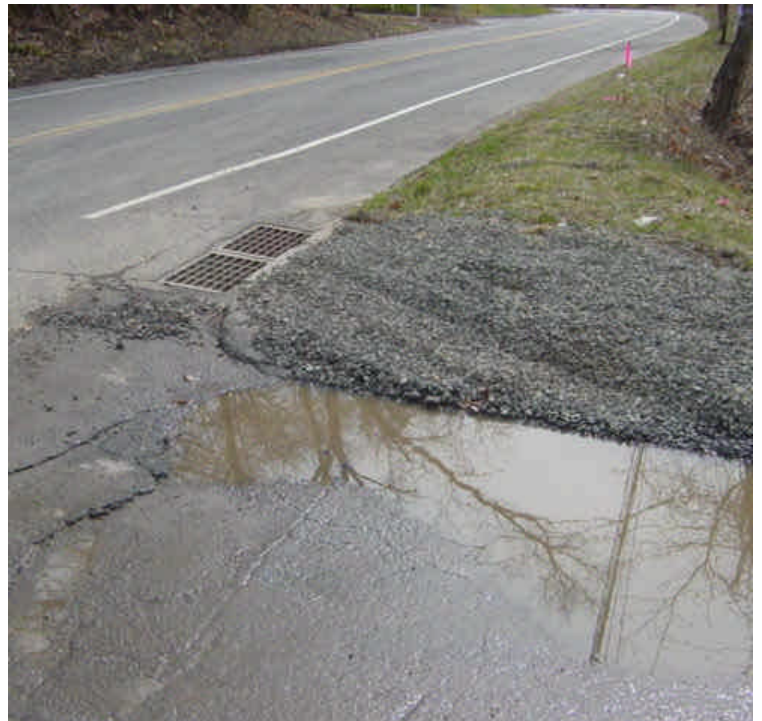
View of the crushed stone in place at the corner of the access drive and Imperial Ave. where the heavy ruts used to be. Ensure that the catch basin here is also protected/controlled.
