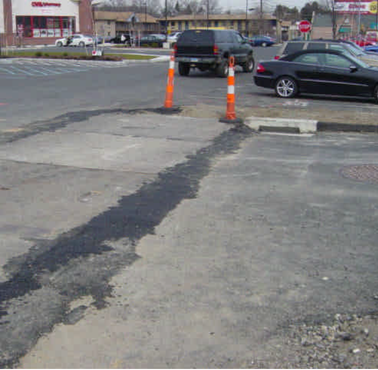
Vault tie-in work continues at sta. #147. The catch basin adjacent to the trench was not protected with controls.
