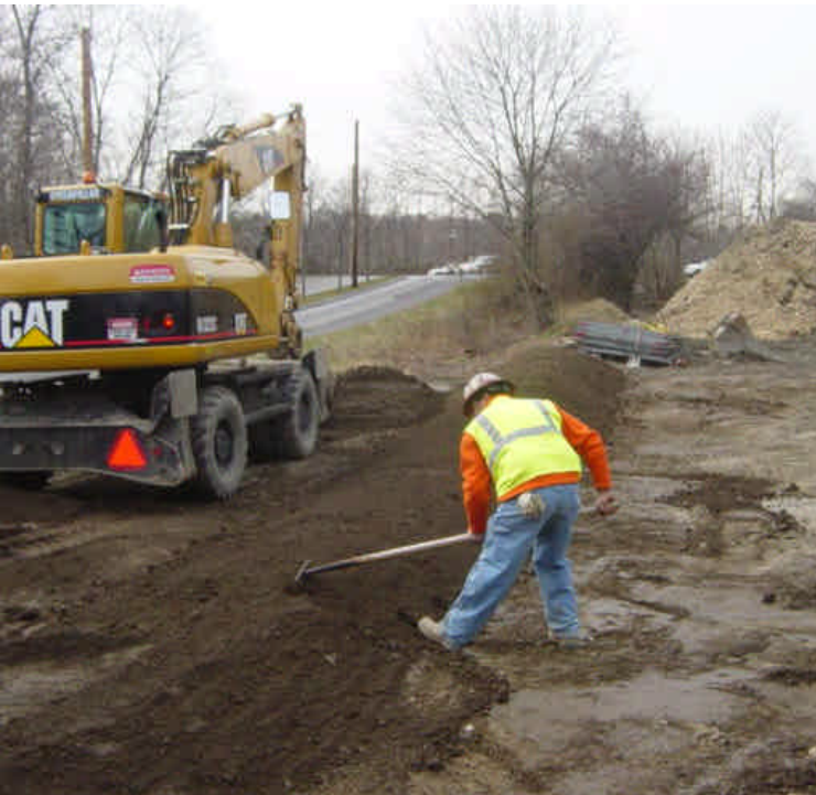
Tie-in work is complete on the east side of the Saugatuck River, near sta. #251. The area is being restored. A dirt berm was being reconstructed near the perimeter of the yard. Ensure that controls are placed adjacent to the berm until the area can re-vegetate.
