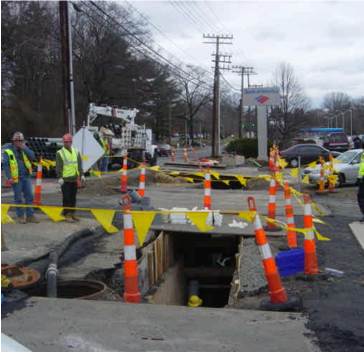
Vault tie-in work continues at sta. #163-166. Conduit was being installed at the time of the inspection. Steel plates remain over portions of the trench.
