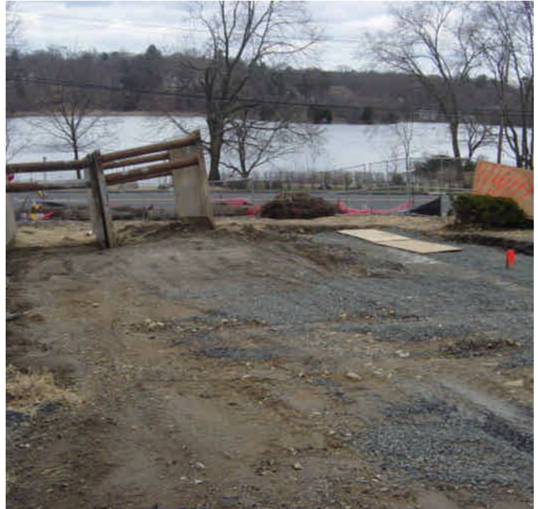
On the west side of the Saugatuck River vault tie-in work is complete and the area has been backfilled. Exposed soil remains stabilized with hay mulch and/or stone. The area is expected to be paved within the next few weeks.
