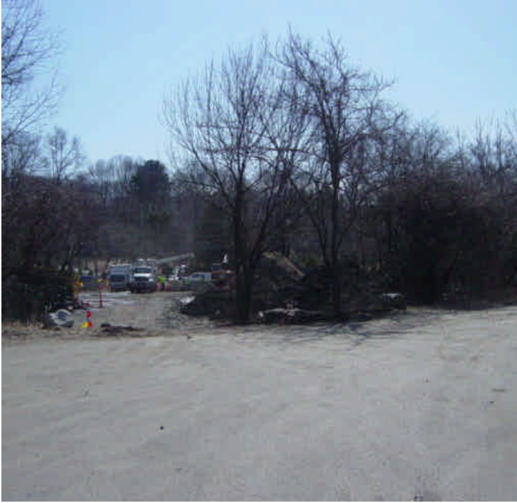
On the east side of the Saugatuck River, vault work continues. Sediment tracking was observed along the parking lot area and the stone construction entrance needs refreshing.
