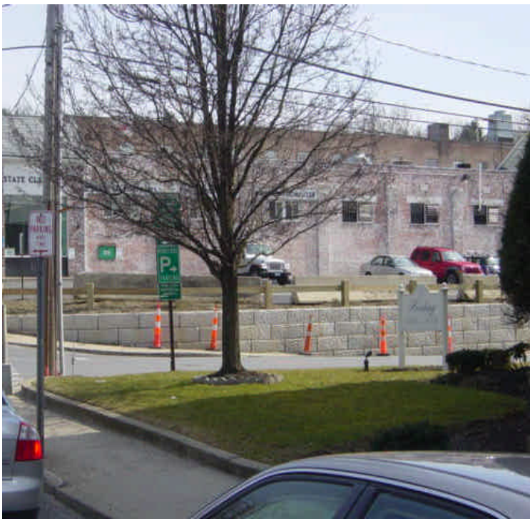
A wooden guide rail has been installed along the top of the retaining wall near sta. #264.
