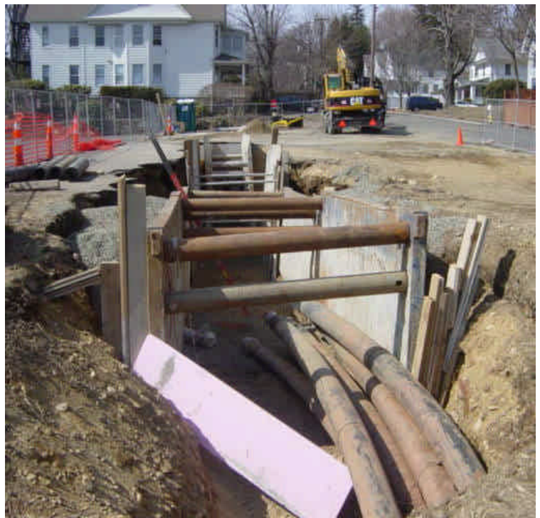
Vault tie-in work continues on the west side of the Saugatuck River near sta. #232. One of the two circuits has already been backfilled.
