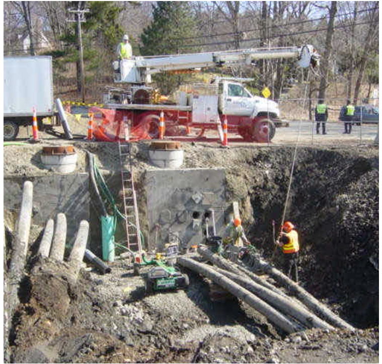
Crews are fusing sections of conduits to complete the tie-in work at the vault near sta. #252.
