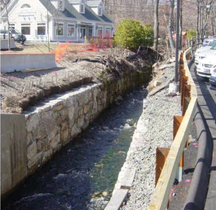
A wooden guide rail has been installed along Stony Brook. Gravel material still appears to have the potential to be washed into the channel. Ensure all material and remaining exposed areas are contained. Consider working with the landowner here to provide shrub plantings for shading.
