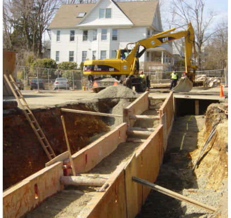
The trench is being backfilled along the west side of the Saugatuck River near sta. #232. The HDD drilling pit remains open.
