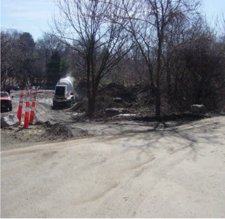
On the east side of the Saugatuck River, vault work continues. Sediment tracking was observed along the parking lot area and the stone construction entrance needs to be refreshed.
