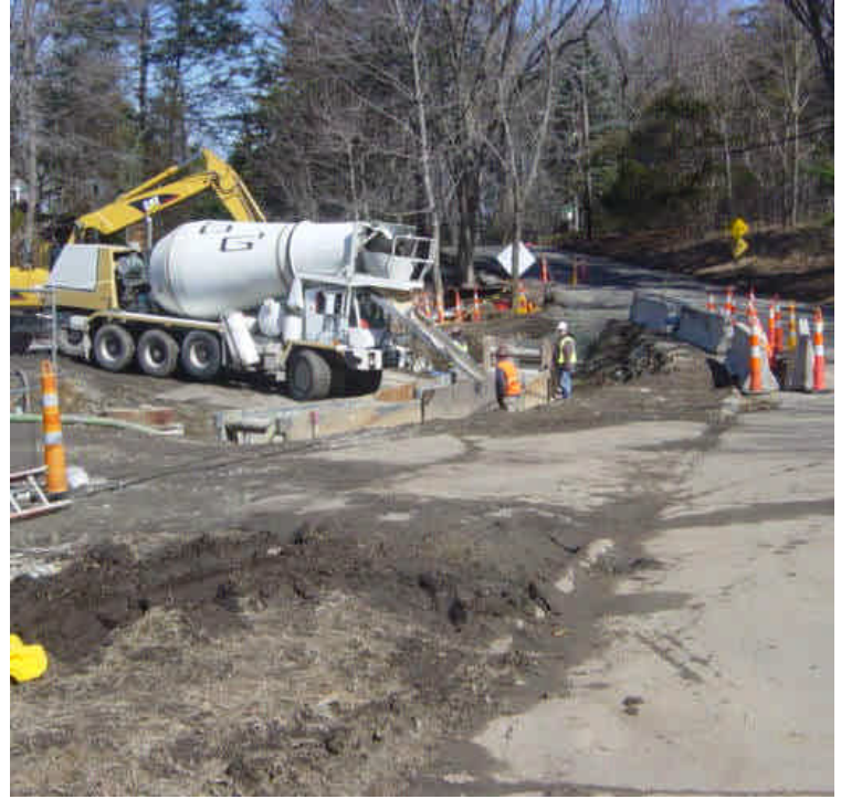
Crews are backfilling the trench near sta. #252 which ties in to the recently installed vault #15.
