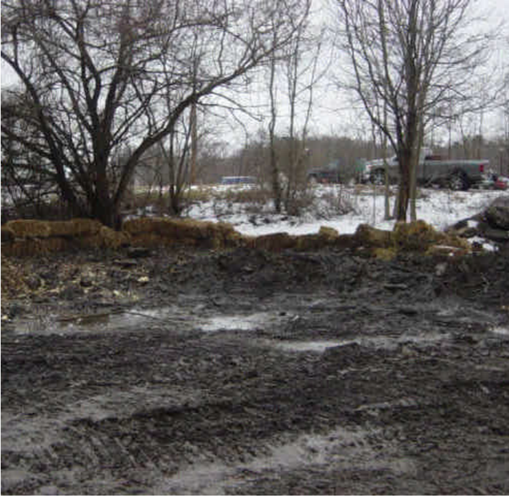
On the east side of the Saugatuck River, excavated soil has been temporarily stockpiled on-site and contained with hay bales. Most of the soil has been transported off site.
