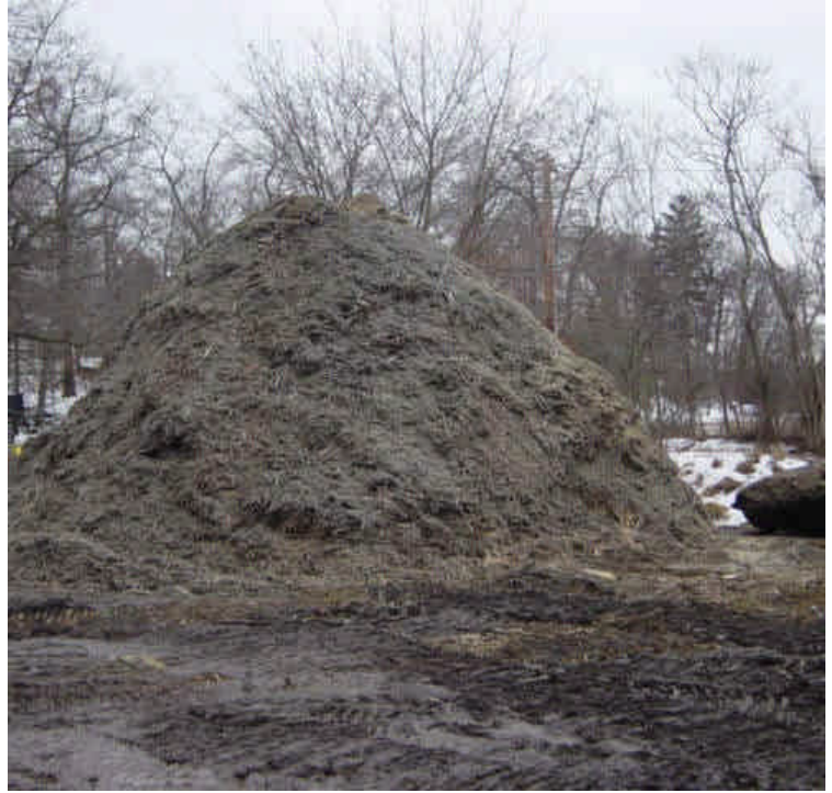
The buried logs that were uncovered during excavation work for vault #15, near sta. #251 have been ground into mulch and stockpiled. A soil stockpile was also noted within the yard.
